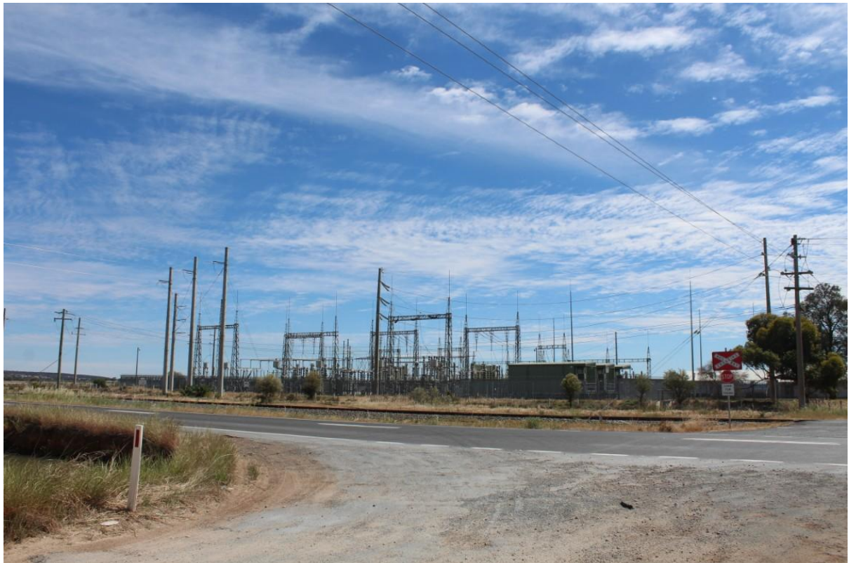
Figure 19 – The Griffith Substation, as viewed from Irrigation Way near the corner of Bob Irvin Road.
