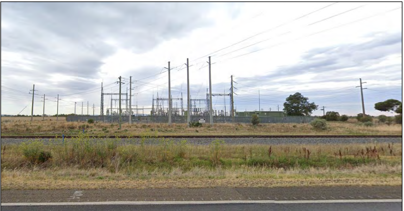
Photo 7: Site conditions of Griffith BESS from Irrigation Way facing north over Griffith Substation with exotic trees. Photo: D.Wall 2024.
