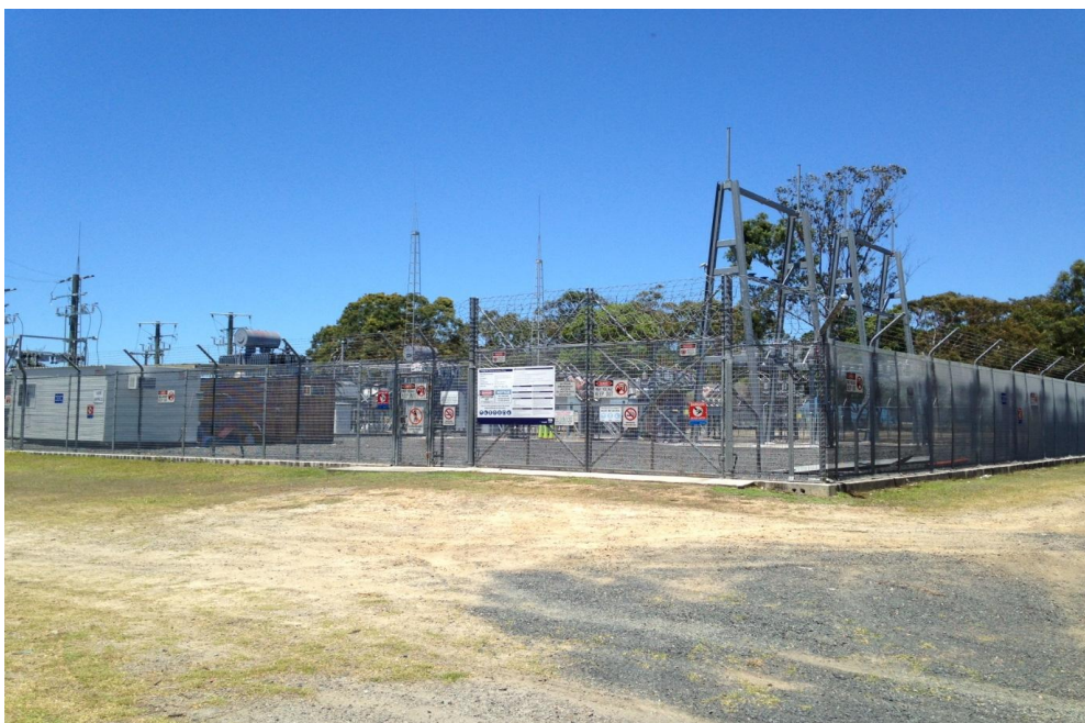
Photo 5 : Vales Point Zone Substation
