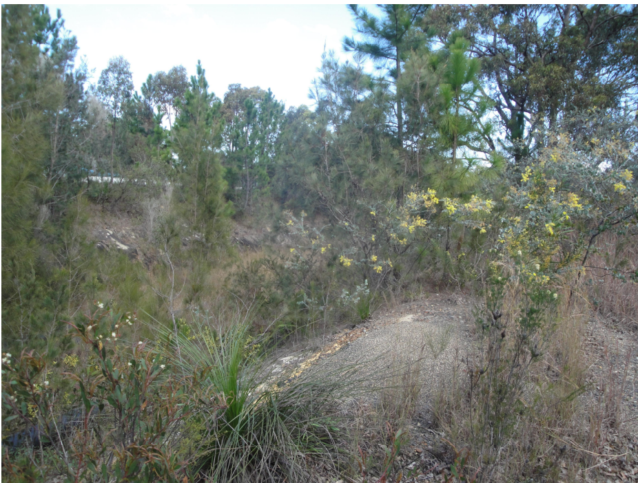
Figure 5.3 : View of the north of assessment area. Conveyor belt construction is accompanied by significant ground disturbance.
