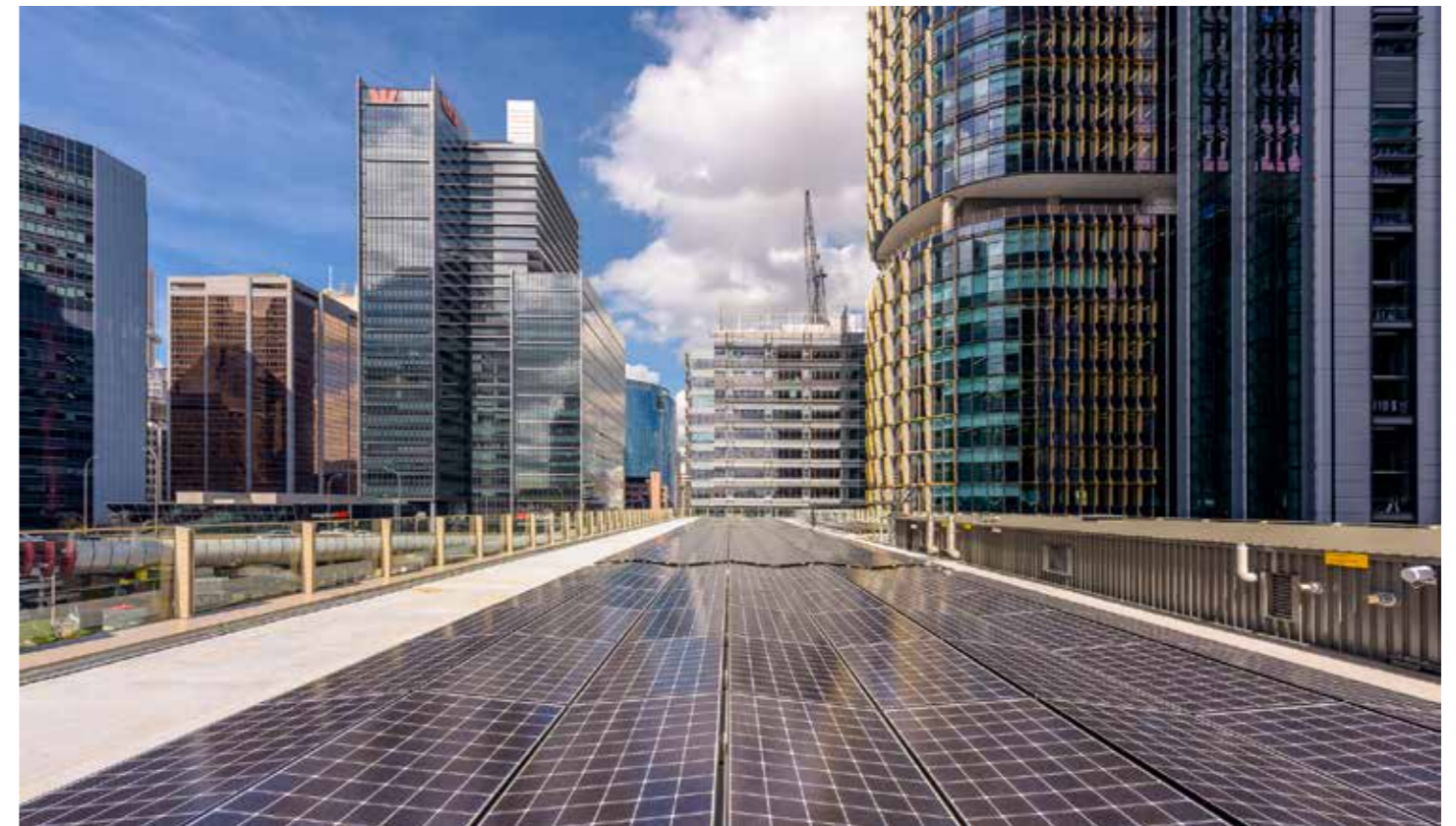
Roof Mounted Photovoltaic Array _ Precedent Commercial Building C2
