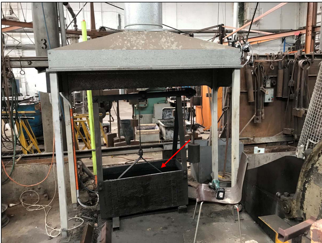
Photograph 8: The oil quenching bath and extraction hood (no walls), located in Bay 2 South.
