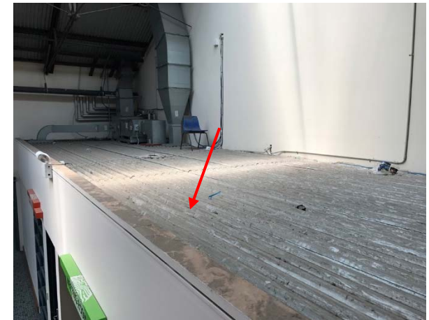
Photo 66: Bay 6 – Lead dust samples collected from the top of the roof of the southern an northern office blocks identified lead contaminated dusts.
