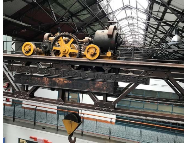
Photo 68: Bay 7 - XRF screening of the overhead travelling crane identified lead based paints. Electrical boards in the operators cabin and brake pads associated with the crane winch gear are presumed to contain asbestos.
