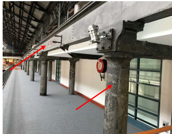
Photo 53: Bay 4 – Structural steel columns, beams and trusses throughout the bay contain lead based paint
