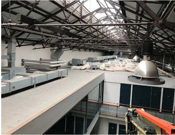
Photo 79: Bay 9 – Lead dust samples collected from the top of the roof of the northern office block identified lead contaminated dusts. XRF screening of heritage structural steel columns, capitals, beams, downpipes, purlins, crane rails and roof trusses throughout the bay identified lead based paints.
