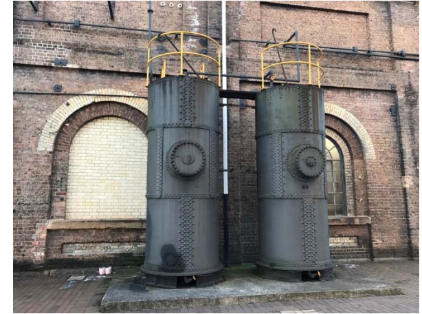
Photo 15: Exterior - Non-rubberised gaskets associated with the pressure vessels at the SE corner of the building contain asbestos
