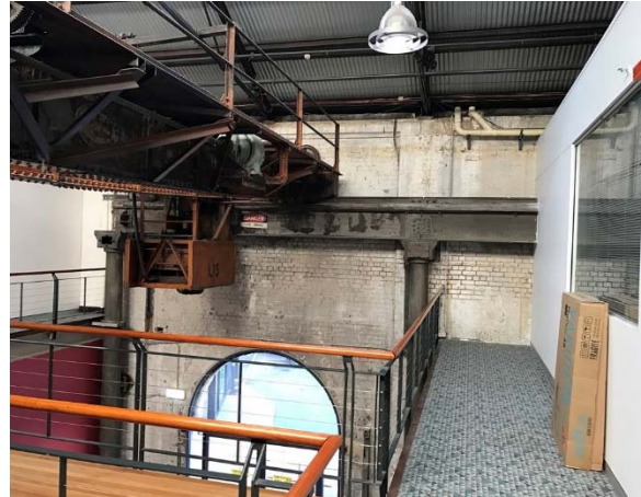
Photo 98: Bay 16 – XRF screening of the overhead travelling crane identified lead based paints. Electrical boards and brake pads associated with the crane are presumed to contain asbestos.
