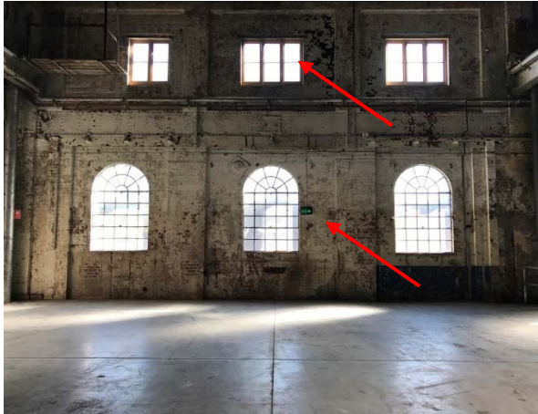
Photo 85: Bays 10 - 14 – All walls, older patchy undercoats concealed beneath the white surface coat may contain lead based paint. XRF screening of the mustard rectangular timber windows located on the upper north and south walls of the bays identified lead based paints.
