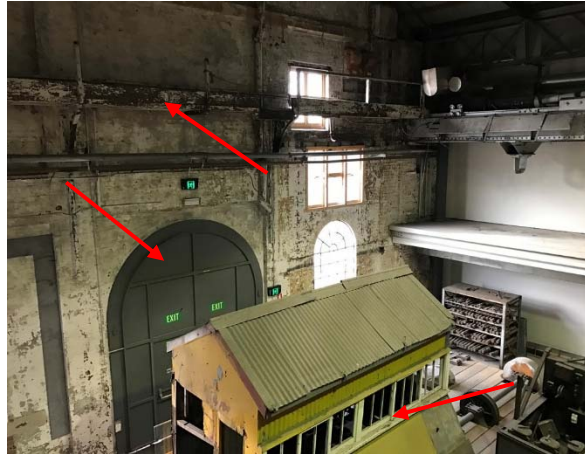
Photo 86: Bays 10 - 14 – XRF screening of the grey metal arched double door located in the bays identified lead based paints. XRF screening of the yellow crane operators cabin in the display area of Bay 10 identified lead based paints.
