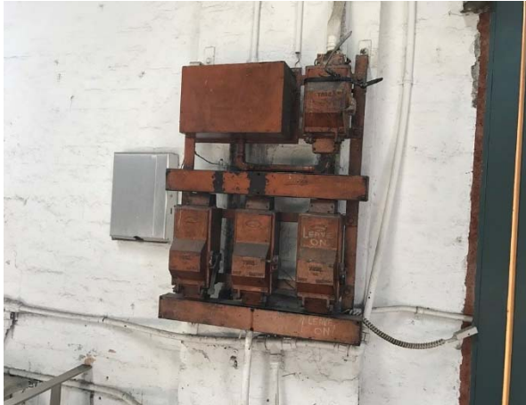
Photo 25: Bay 1 north - Fuse box compartments on north wall contain asbestos paper linings (friable)
