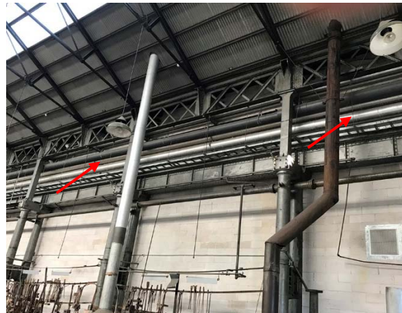
Photo 47: Bay 2 - Old pipework associated with the former steam plant may contain asbestos gaskets. Old and new pipework traversing the upper walls of the bay is insulated with SMF
