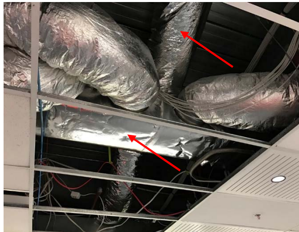
Photo 77: Bay 9 – Fixed and flexible air-conditioning ductwork within office ceiling cavities is insulated with SMF.
