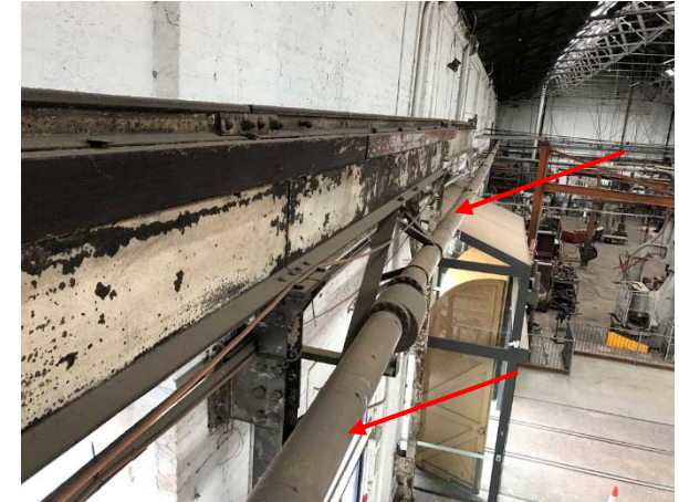
Photo 39: Bay 1 – Old pipework associated with the former steam plant may contain asbestos gaskets. Old and new pipework traversing the upper walls of the bay is insulated with SMF
