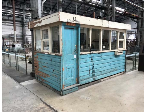
Photo 38: Bay 1 north - XRF screening of the blue Sub Foreman's Office identified lead based paint.
