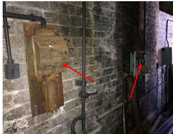
Photo 11: Exterior – SE Annex & Boiler House, XRF screening of old electrical boxes identified lead based paint. Potential ACM may be present in boxes that could not be opened at the time of inspection.
