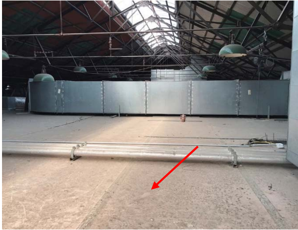
Photo 61: Bay 5 south – A lead dust sample collected from the top of the southern theatre identified lead contaminated dusts. Fixed and flexible air-conditioning ductwork is insulated with SMF.
