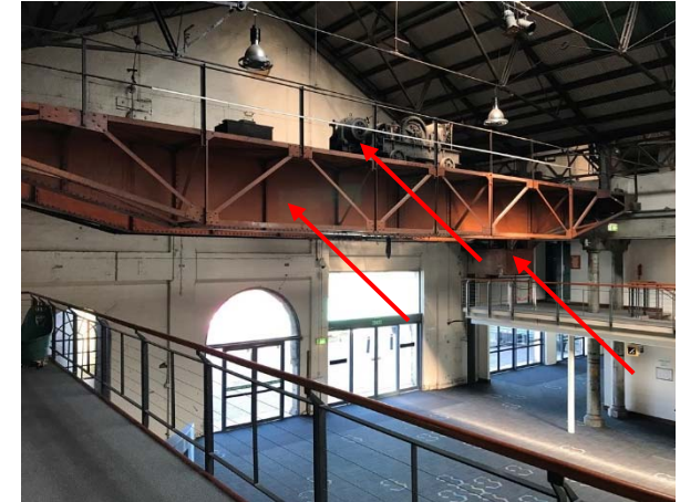
Photo 51: Bay 4 south - XRF screening of both overhead travelling cranes in the bay identified lead based paints. Electrical boards in the operators cabins and brake pads associated with the crane winch gear are presumed to contain asbestos.
