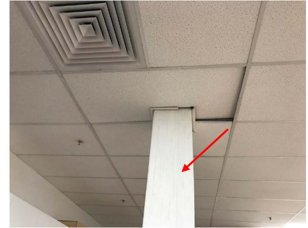
Photo 63: Bay 6 south - XRF screening of the square timber columns and beams in the working space and ceiling cavity identified lead based paint
