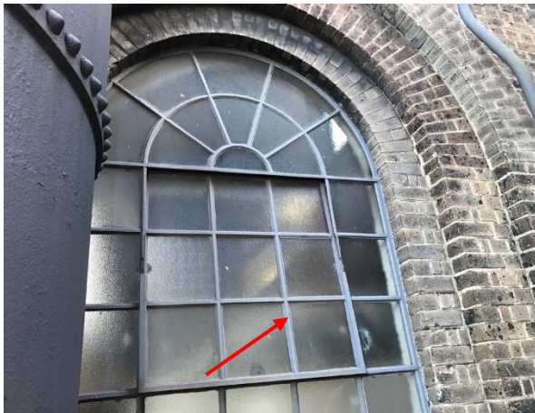
Photo 22: Exterior – Bay 4 south, XRF screening of the heritage arched window identified lead based paint
