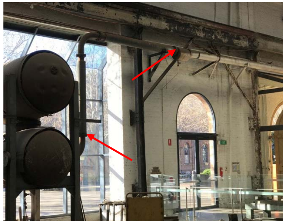
Photo 29: Bay 1 - Non-rubberised gaskets associated with the Davy water feed pipe contain asbestos based gaskets
