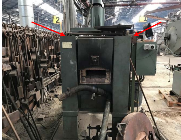
Photo 26: Bay 1 south - The top seal on the HC Thornthwaite Furnace is woven asbestos (friable)
