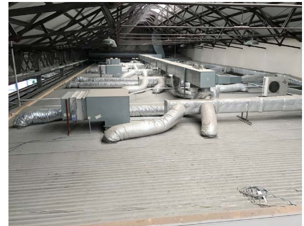
Photo 78: Bay 9 – Lead dust samples collected from the top of the roof of the southern office block identified lead contaminated dusts. Fixed and flexible air-conditioning ductwork on the Level 1 office roof is insulated with SMF.
