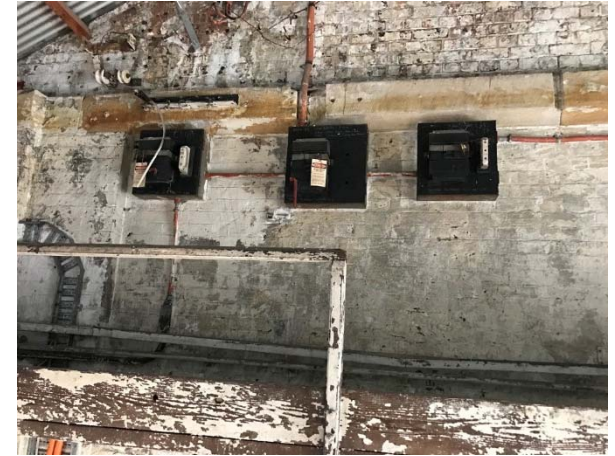
Photo 81: Bay 10 north - Three black electrical boards on the upper north wall of Bay 10 are presumed to contain asbestos
