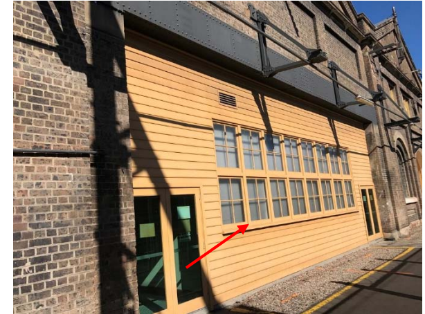
Photo 21: Exterior – Bay 8 north, XRF screening of the older mustard coloured timber window frames identified lead based paint. XRF screening of newer timber panelling did not identify lead based paint
