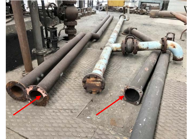
Photo 27: Bay 1 north - Residual gaskets on old pipes on the floor of the Davy display contain asbestos. Several of these gaskets are in poor condition and should be removed.
