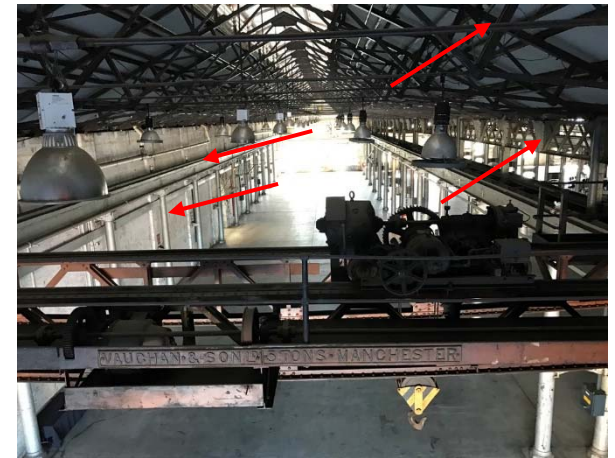
Photo 84: Bays 10 - 14 – XRF screening of heritage structural steel columns, capitals, beams, downpipes, purlins, crane rails and roof trusses throughout the bay identified lead based paints
