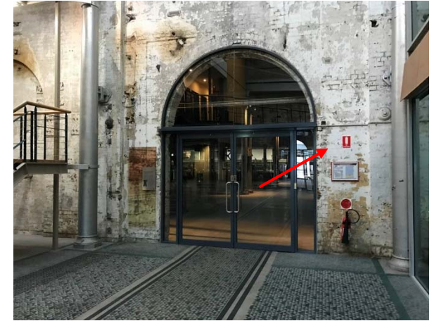
Photo 93: Bay 15 – XRF screening of off-white paint on the eastern wall adjacent the Central Road access door identified lead based paints. A black undercoat was observed in this location.
