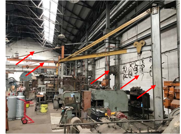
Photo 45: Bay 2 - XRF screening of the jib cranes and electrical boxes identified lead based paint. Lead based undercoat paints may be present beneath the white perimeter walls of Bay 2.
