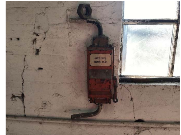
Photo 30: Bay 1 north - Control relay box compartments on north wall contain asbestos paper linings (friable)
