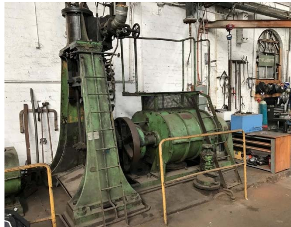
Photo 35: Bay 1 south - The green Blower No.6 contains lead based paint
