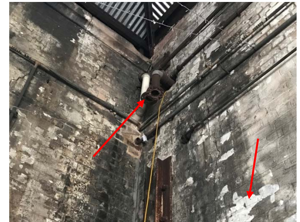
Photo 6: Exterior – SE Annex, suspected asbestos containing gaskets and potential lead based paint
