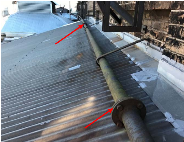
Photo 7: Exterior, SE Annex - Non-rubberised gaskets associated with the water pipe traversing the awning are assumed to contain asbestos.
