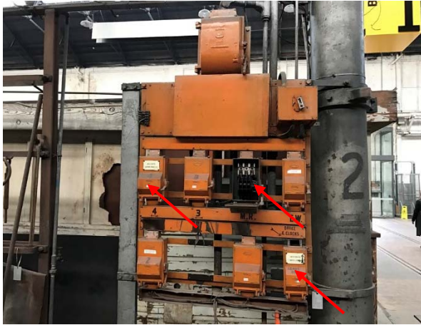
Photo 43: Bay 2 north - Fuse box compartments in the SE of Bay 2 south contain asbestos paper linings (friable)
