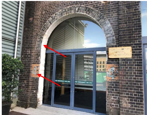
Photo 17: Exterior – North & south walls, XRF screening of residual white paint around brick archways and old orange and white bay number signs identified lead based paint
