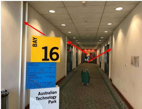
Photo 100: Bay 16 – XRF screening of the white RSJ stanchions in the ground level central hallway of Bay 16 south identified lead based paint
