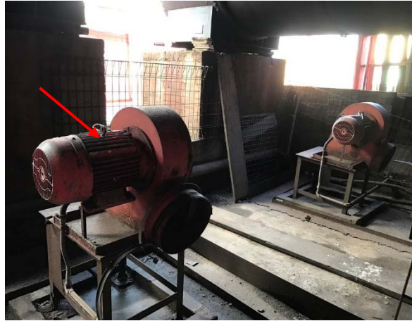
Photo 14: Exterior – Boiler House, XRF screening of the orange boiler gaskets identified lead based paint
