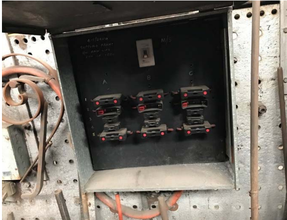
Photo 31: Bay 1 south - Two old black electrical board in the central west of Bay 1 south are presumed to contain asbestos
