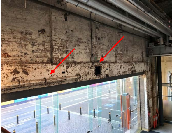
Photo 73: Bay 8 – Lead dust samples collected from the top of the lintel beam above the southern entry doors identified lead contaminated dusts. The off-white paint on the lintel beam is lead based paint.
