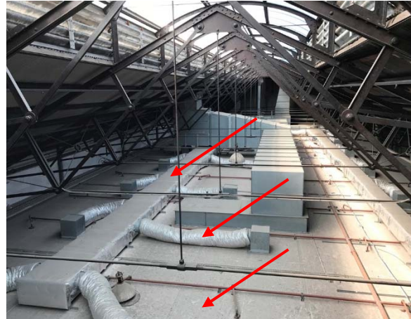
Photo 50: Bay 3 south – A lead dust sample collected from the top of the southern function centre identified lead contaminated dusts. Fixed and flexible air-conditioning ductwork is insulated with SMF.
