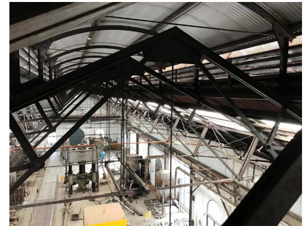
Photo 36: Bay 1 - XRF screening of heritage structural steel columns, capitals, beams, downpipes, purlins, crane rails and roof trusses throughout the bay identified lead based paint
