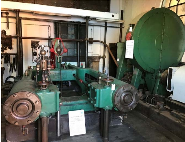
Photo 49: Bay 3 south, Pump House – The green Fielding & Platt steam and electric pumps in the southern Pump House annex, contain lead based paint
