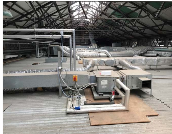
Photo 71: Bay 7 – Lead dust samples collected from the top of the roof of the northern office block identified lead contaminated dusts.
