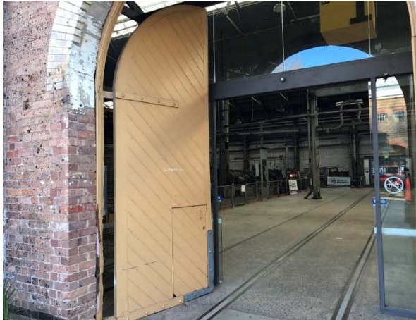
Photo 19: Exterior – East wall, XRF screening of the mustard coloured central door identified lead based paint
