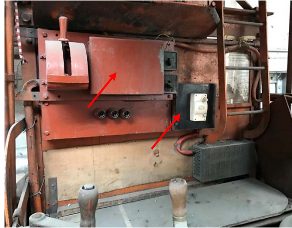
Photo 56: Bay 5 - Electrical boards in the operators cabin overhead crane are presumed to contain asbestos.
