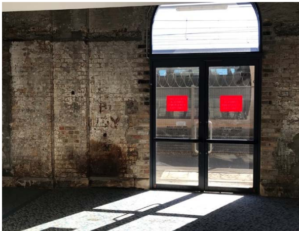
Photo 52: Bay 4 north – Residual paints on the northern wall of the bay are lead based paint. Lead based undercoat paints may be present beneath the white perimeter walls in other areas.
