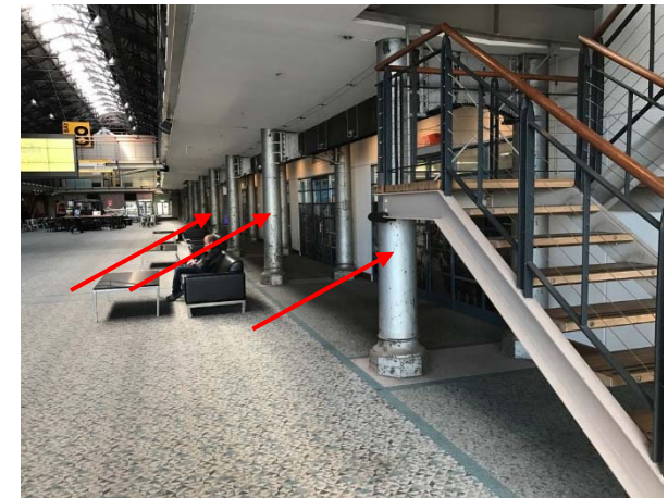
Photo 72: Bay 8 - XRF screening of heritage structural steel columns, capitals, beams, downpipes, purlins, crane rails and roof trusses throughout the bay identified lead based paint
