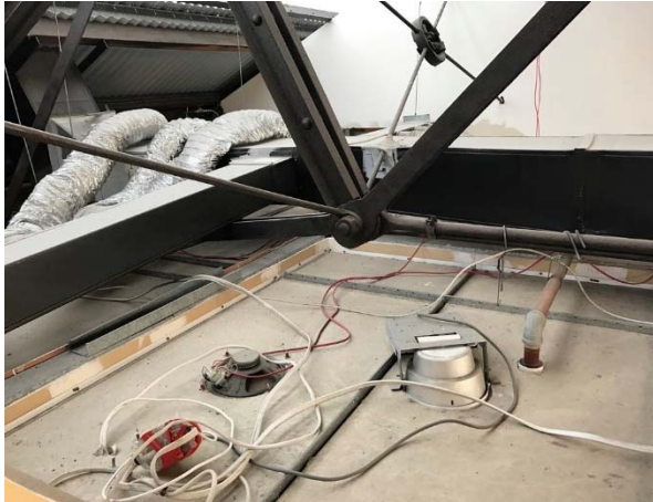
Photo 97: Bay 15 – A lead dust sample collected from the flat roof of the northern office amenities area identified lead contaminated dusts.
