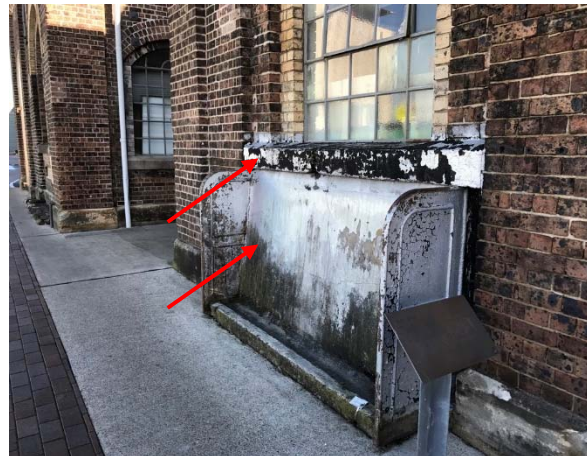
Photo 23: Exterior – Bay 9 south, XRF screening of the silver external urinal and overlying window sill identified lead based paint
