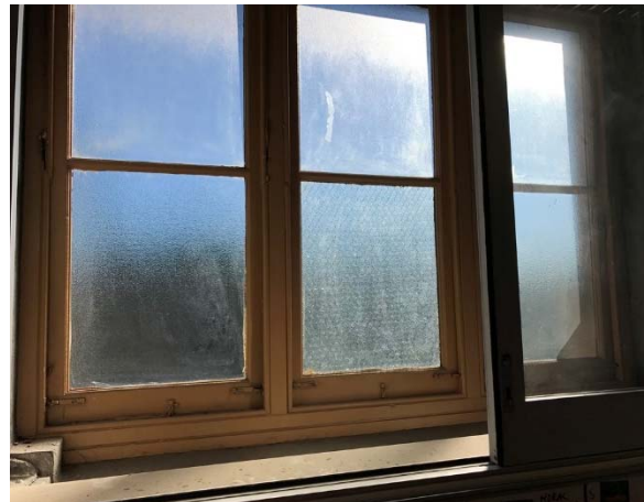
Photo 101: Bay 16 – XRF screening of the mustard coloured rectangular timber windows on Level 1 identified lead based paint
