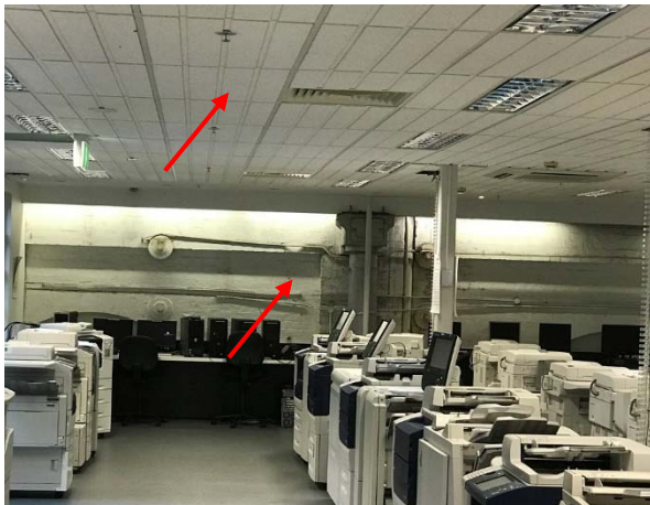
Photo 58: Bay 5 – All walls, older patchy undercoats concealed beneath the white surface coat may contain lead based paint. Ceiling tiles contain SMF.
