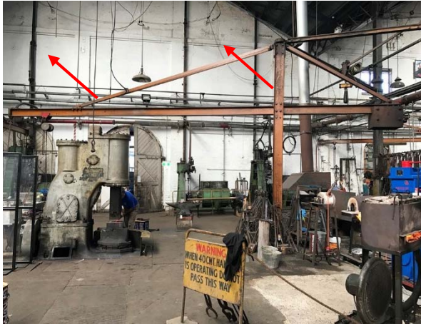
Photo 37: Bays 1 & 2 – All walls, older patchy undercoats concealed beneath the white surface coat may contain lead based paint
