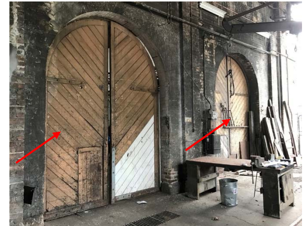
Photo 9: Exterior – SE Annex, mustard coloured timber double arched door at south of Bay 1 contain lead based paint. Flaking paint should be removed and managed.
