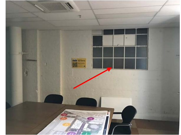
Photo 69: Bay 7 – XRF screening of the off-white heritage arched window on the southern wall identified lead based paint
