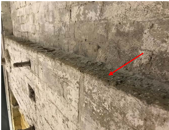
Photo 88: Bay 11 – A lead dust sample collected from the upper northern wall ledge of Bay 11 identified lead contaminated dusts. Accumulated dust and debris is typical on upper wall ledged throughout Bays 10 - 14.
