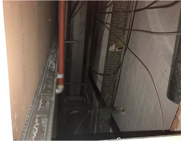
Photo 62: Bay 5 south – Dusts concealed in wall cavities / plenums of Bay 5 and Bay 6 south may be lead impacted. These areas should be assessed prior to demolition.
