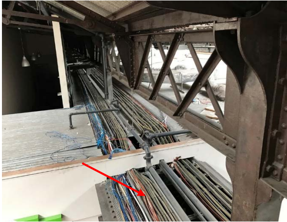
Photo 67: Bay 6 – A lead dust swab sample collected from the top of the cable tray above Central Road identified lead contaminated dusts.
