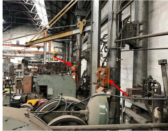
Photo 44: Bay 2 - Several electrical boxes in Bay 2 contain backing boards assumed to contain asbestos. Some of the boxes could not be opened at the time of inspection
