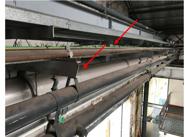
Photo 75: Bay 8 – Lead dust samples collected from the top of the cable tray above the southern entry doors identified lead contaminated dusts. Pipework traversing the upper north and south walls are insulated with SMF.
