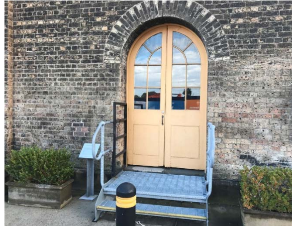
Photo 20: Exterior – Bay 3 south wall, XRF screening of the mustard coloured timber arched doors identified lead based paint
