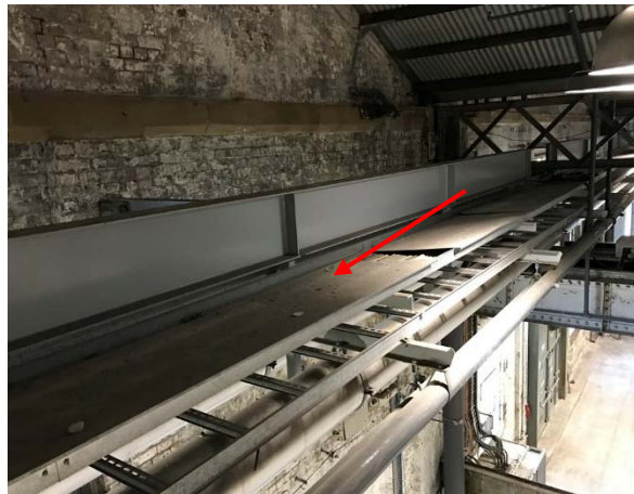
Photo 89: Bay 13 – A lead dust sample collected from the main cable tray above the upper southern wall of Bay 13 identified lead contaminated dusts. This cable tray traverses Bays 10 - 14.
