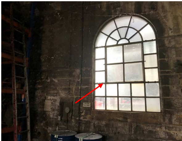
Photo 10: Exterior – SE Annex, arched heritage window frame on west wall contains lead based paint. Flaking paint should be removed and managed.
