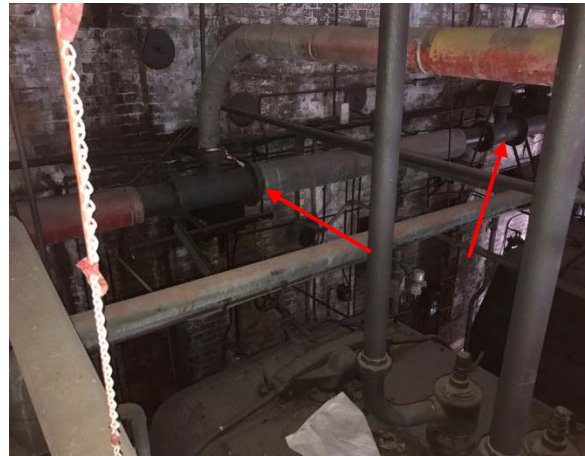
Photo 8: Exterior – Boiler House, old, unrestored boiler pipework assumed to contain asbestos gaskets
