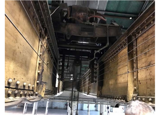
Photo 87: Bays 10 - 14 – XRF screening of overhead travelling cranes located in the bays identified lead based paints
