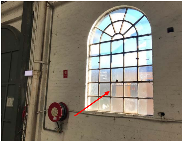
Photo 46: Bay 2 north - XRF screening of the heritage arched window frame on the northern wall identified lead based paint
