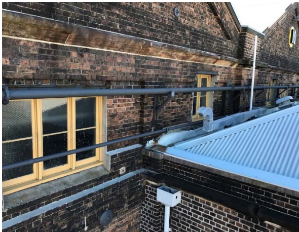
Photo 16: Exterior – XRF screening of the mustard coloured timber rectangular windows in the upper north, south and west walls identified lead based paint
