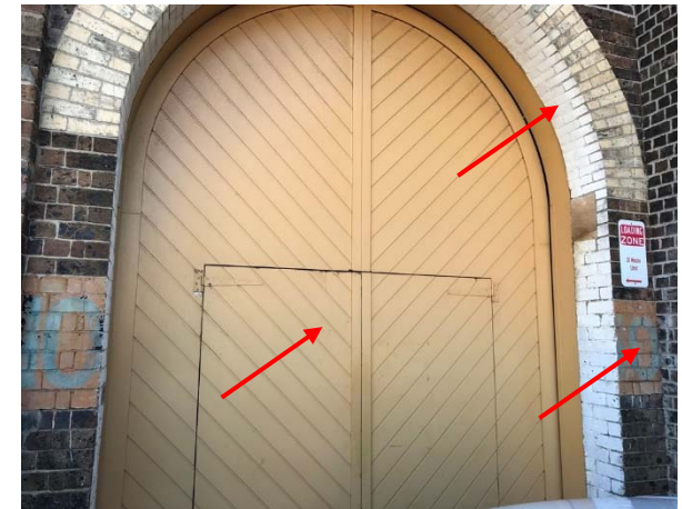
Photo 18: Exterior – XRF screening of 'original' mustard coloured timber double arched doors identified lead based paint. Newer western red cedar replacement doors do not contain lead based paint.
