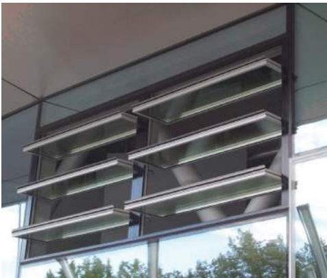
Actuated glass smoke ventilation louvres
