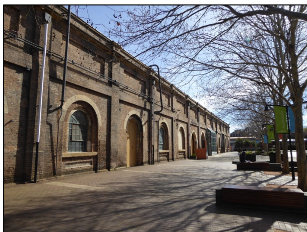
FIGURE 85: VIEW NORTH ALONG EASTERN FAÇADE OF LOCOMOTIVE WORKSHOP, EXAMPLE OF BRICKED OVER HERITAGE WINDOW TO BE RESTORED FOURTH OPENING TO RIGHT IN IMAGE (SOURCE: CURIO 2016)
