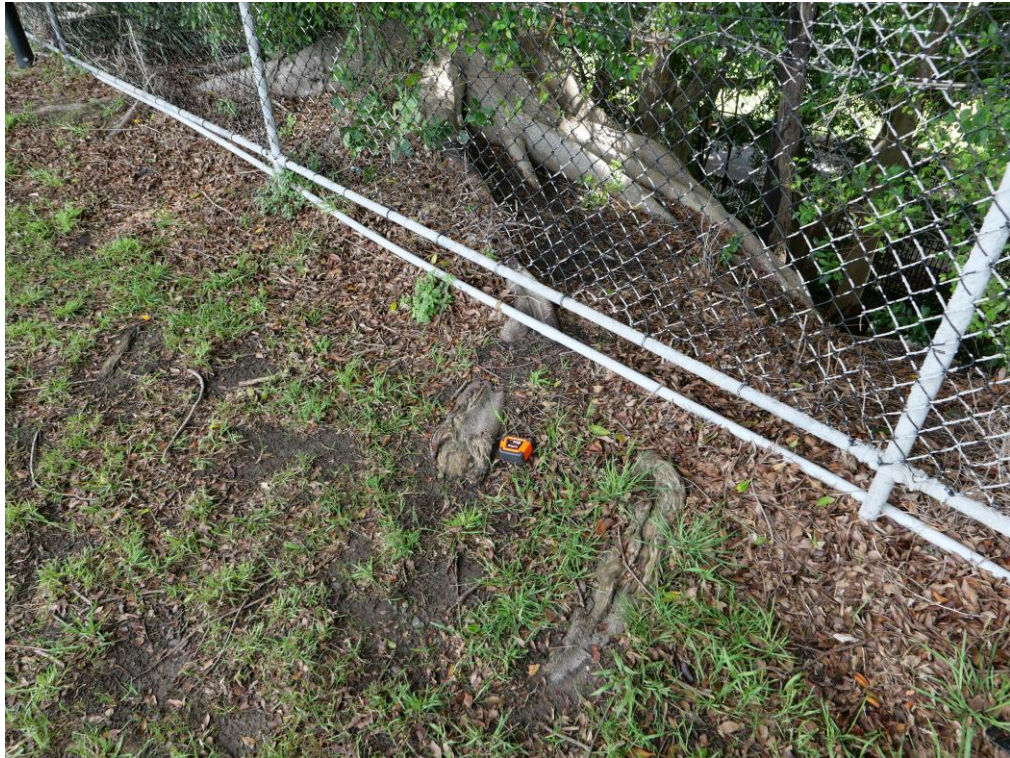
Plate 4 – showing some roots ascending up into the lawn terrace.
