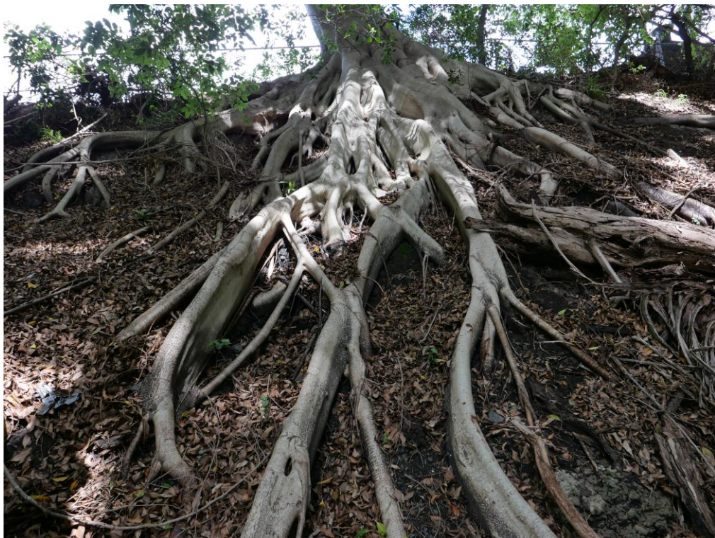
Plate 3 – showing network of woody surface roots extending down the embankment
