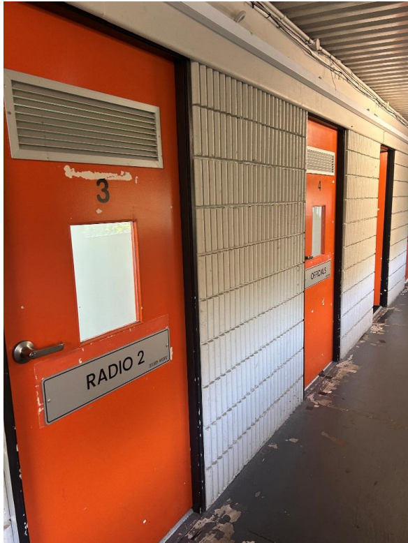
Figure 45: Upper level radio rooms
