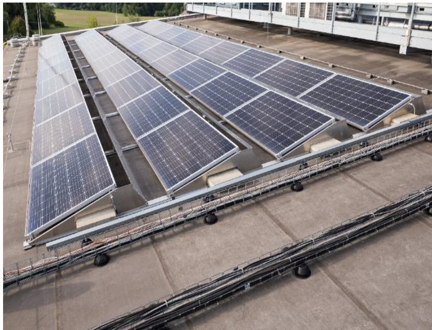
Figure 10 Example of rooftop solar installation
