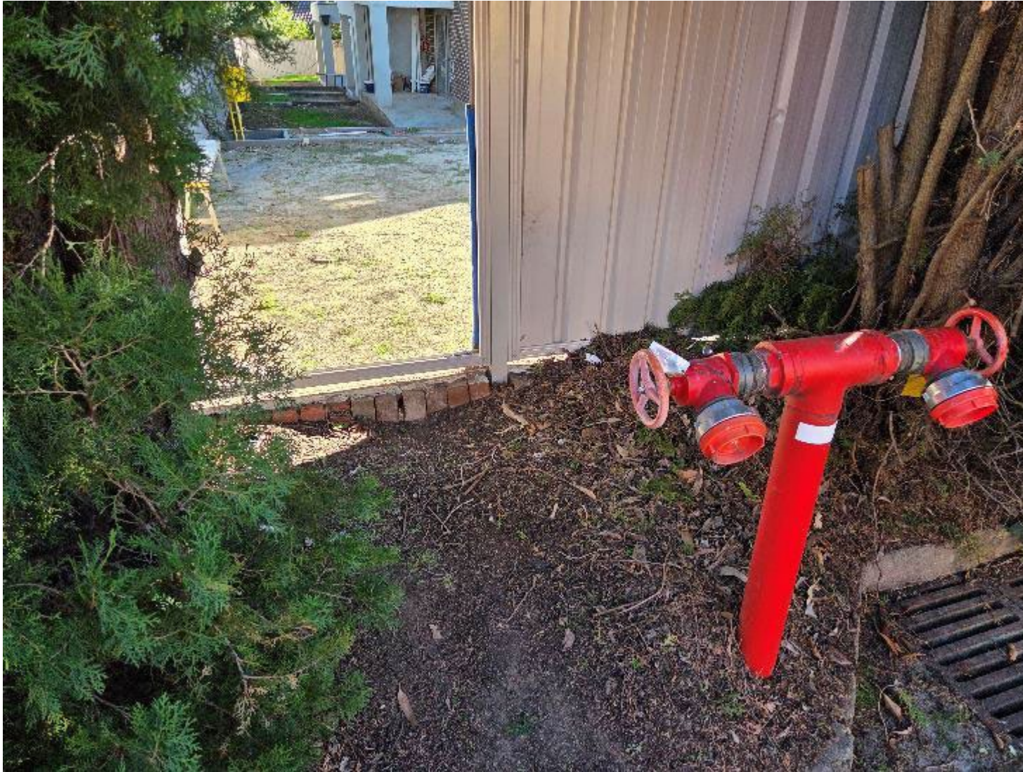
Fig. 74 Photo of water mains and stormwater between T57 & T58.
