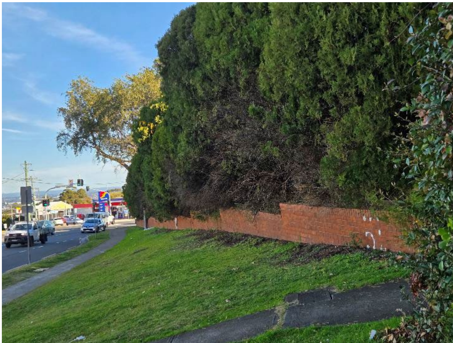
Fig. 100. Photo facing South showing a brick retaining wall along the road frontage to Pennant Hills Road where trees have been planted adjacent to the wall and will have formed an asymmetric root plate.
