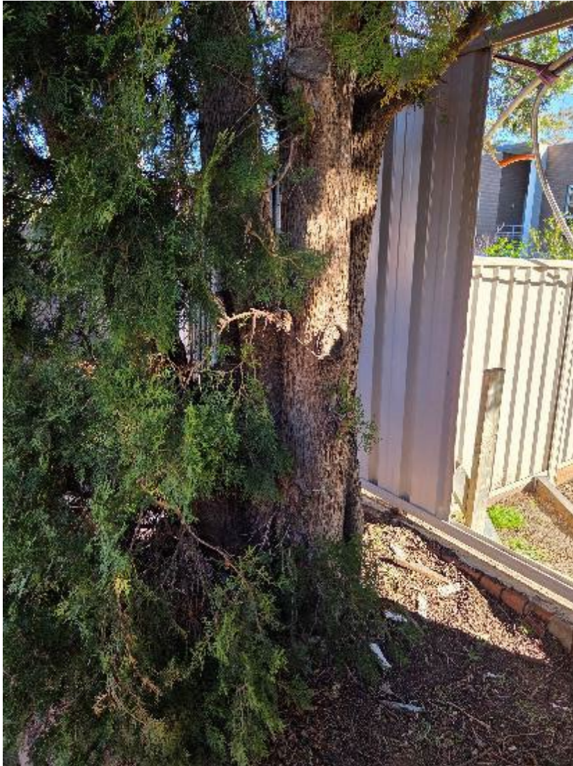
Fig. 72. Photo of T58 showing co dominant stems which adjoin in 'V' Shaped stem unions at the base of the tree.
