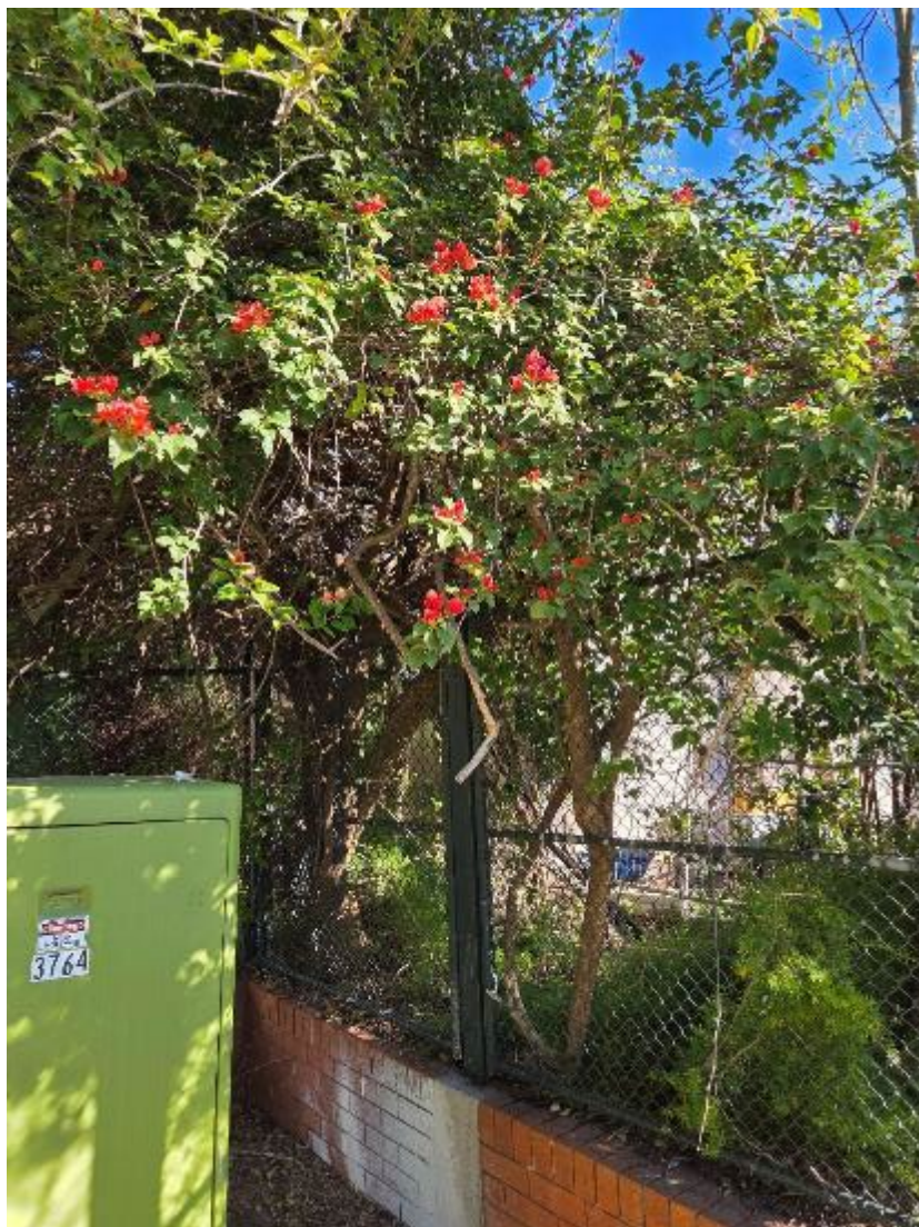
Fig. 95. Photo showing Bouganvillea vines surrounding the electrical substation in the Northwest portion of the Site.
