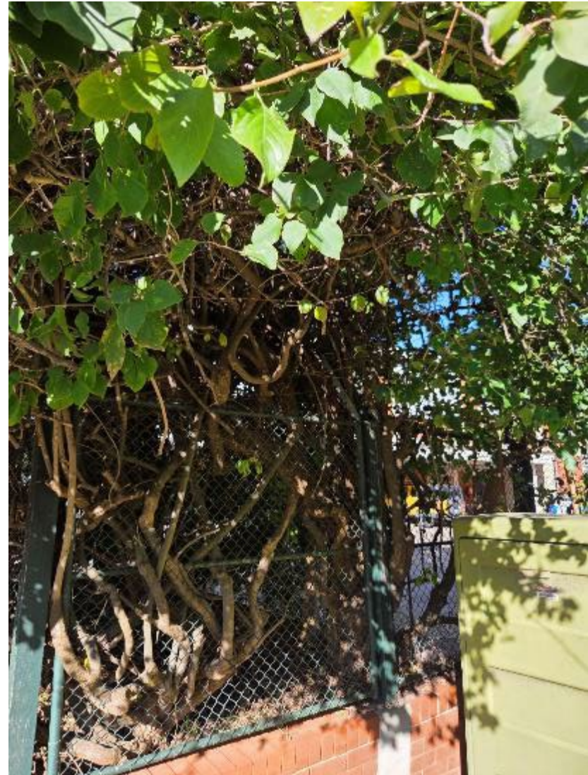
Fig. 94. Photo showing Bougainvillea vine surrounding the electrical substation in the Northwest portion of the Site.
