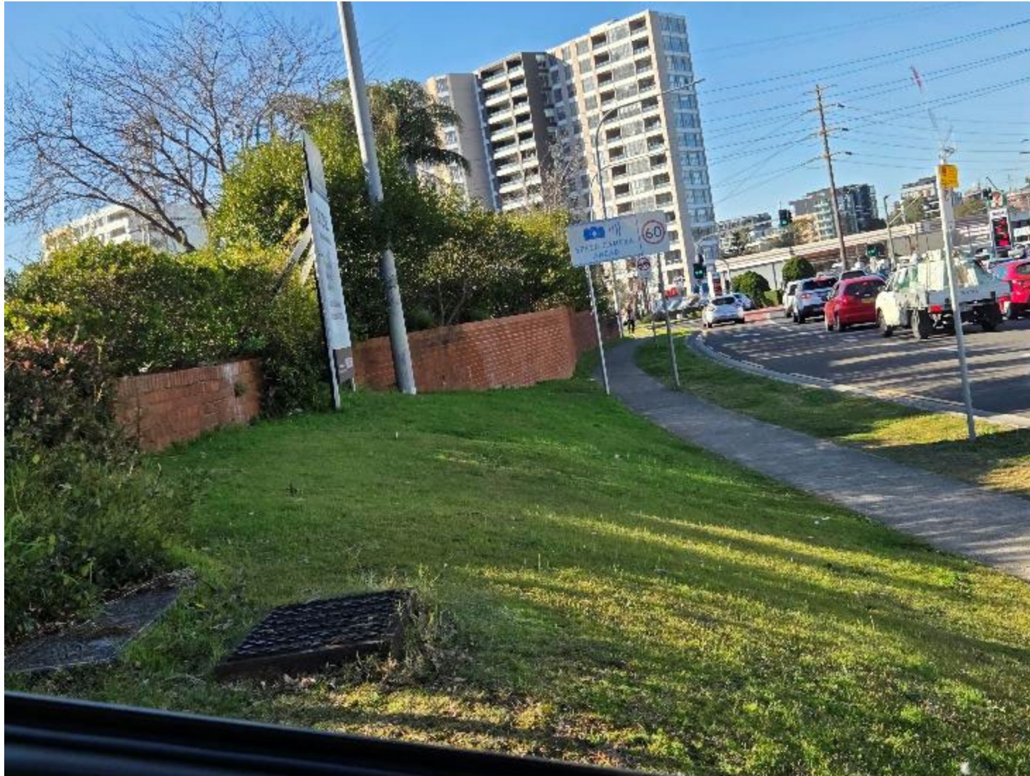
Fig. 101. Photo facing North showing a brick retaining wall along the road frontage to Pennant Hills Road where trees have been planted adjacent to the wall and will have formed an asymmetric root plate.
