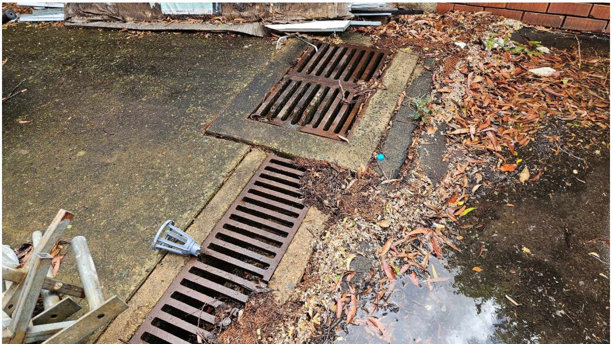
Plate 10. Deep drainage system present in the west of the Project Area, with grating covering the drain. (Source: Heritage Now 2024)
