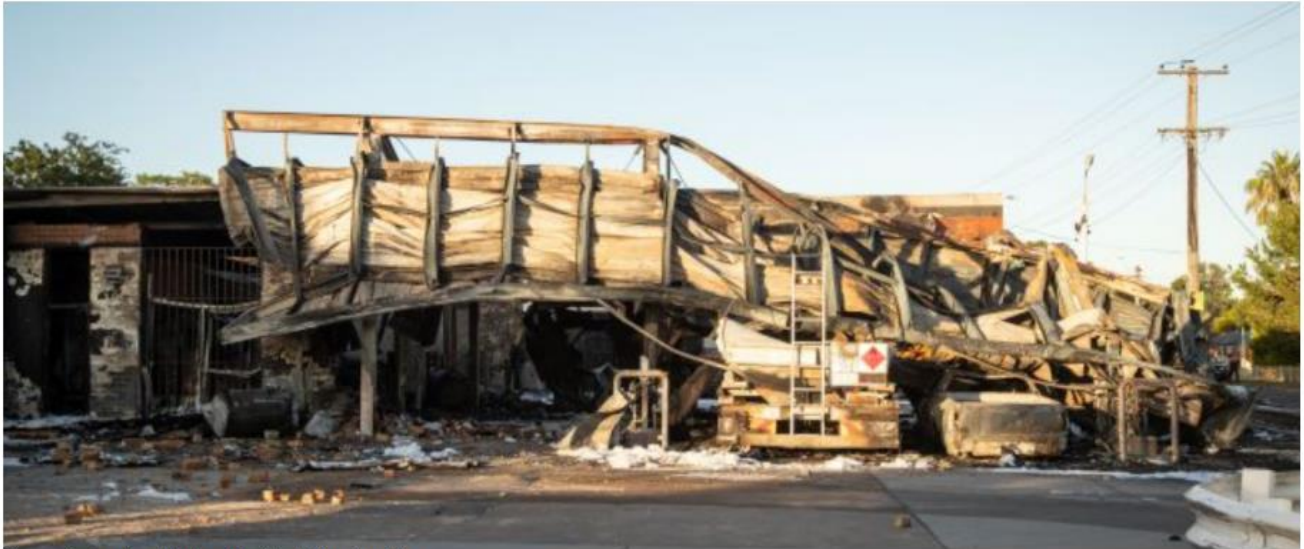
Figure 4: Service Station Facility Following Fire
