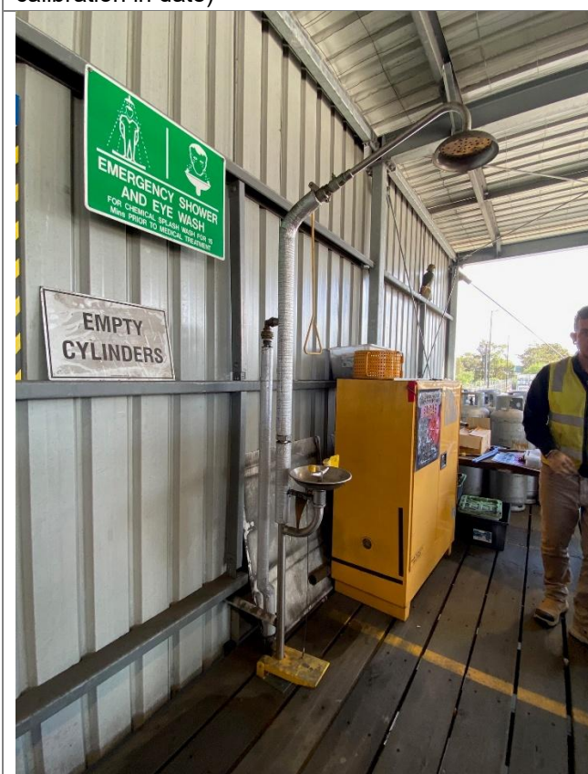
Photo 9: Emergency shower and eyewash station in the cylinder filling area
