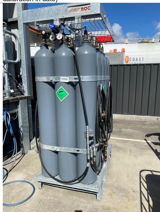
Photo 10: Compressed nitrogen storage adjacent to the cylinder filling area
