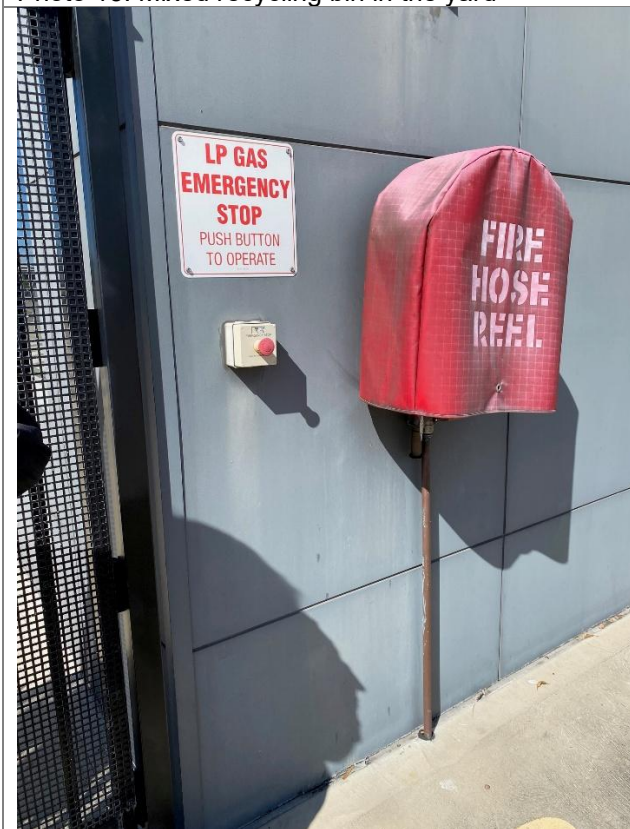
Photo 17: Emergency stop and fire equipment near the bulk LPG tank
