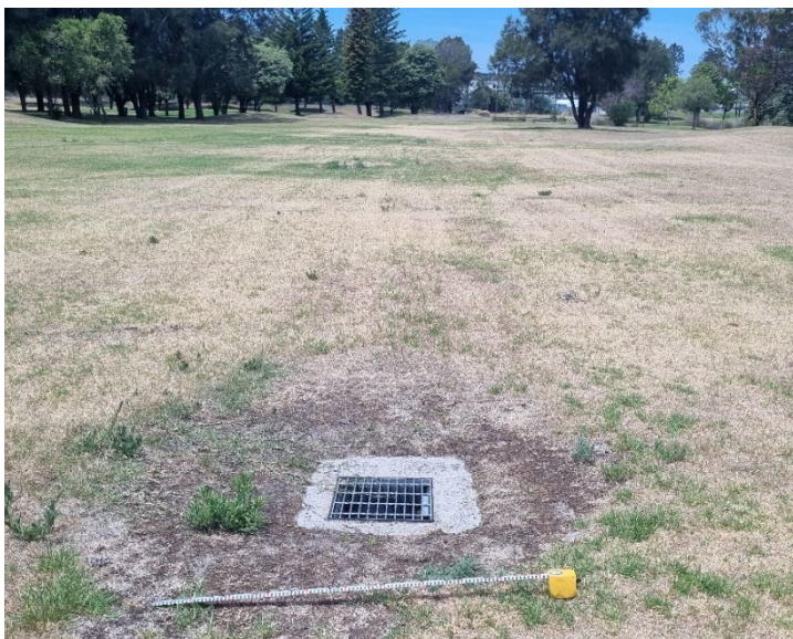
Photo 14 An example of high GSV (80%+) adjacent to subsurface utilities services, facing north
