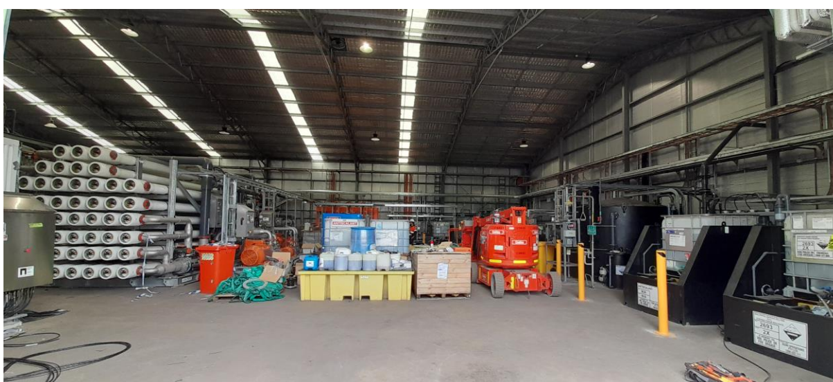
Photo 1: Internal of the WTP Shed, Reverse Osmosis (RO) skid installed, chemical storage (right)
