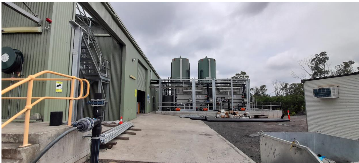
Photo 3: External of the WTP shed, SUF tanks in the centre of picture
