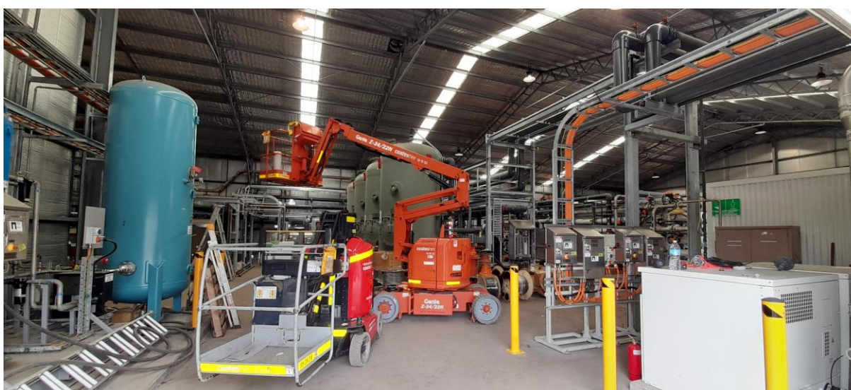
Photo 2: Internal of the WTP Shed, Ion Exchange
