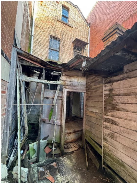
Figure 14: Dilapidated shed at rear of 265 Pacific Highway.
