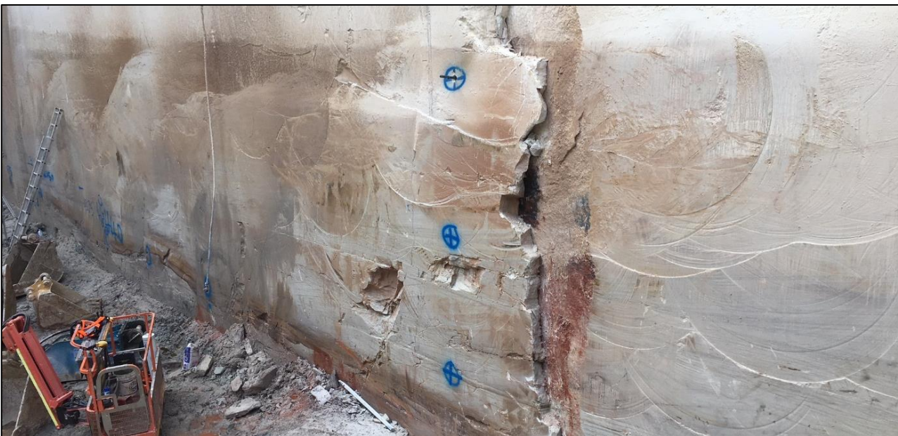
Figure 1: Example 'feathered edge' in Sandstone excavation sidewall
