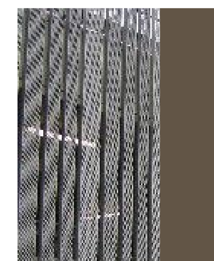
6 - LOUVRES - CAR PARK
