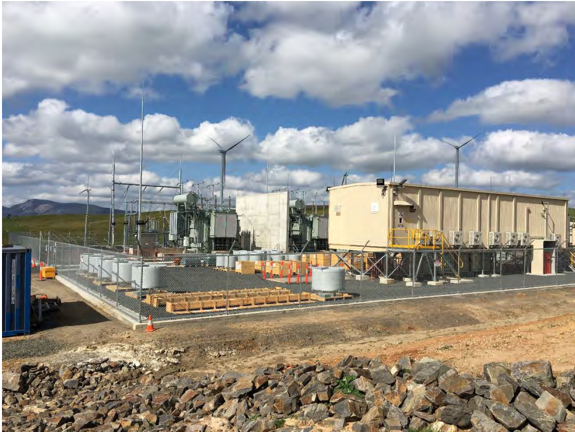
d) Example of a substation
