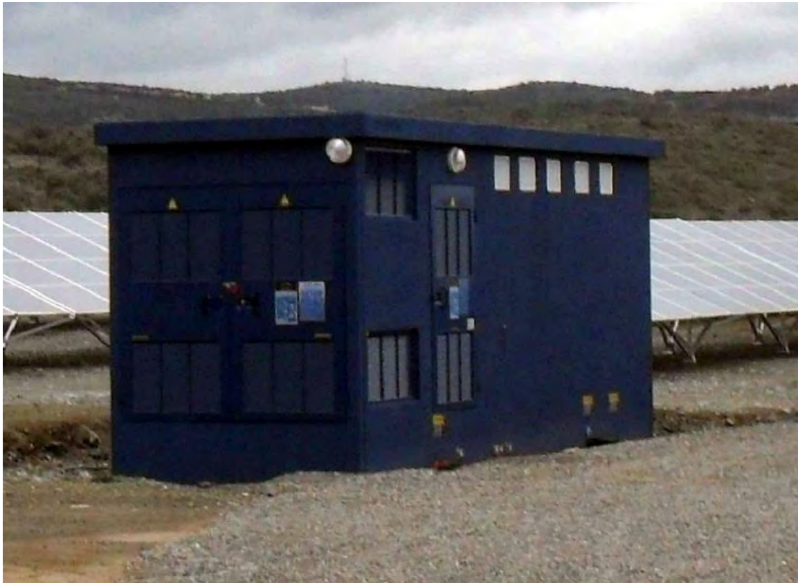
b) Example of a power conversion unit
