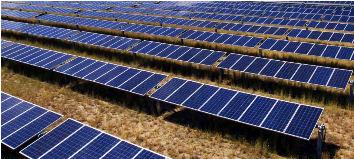
a) Solar arrays single axis tracking system
