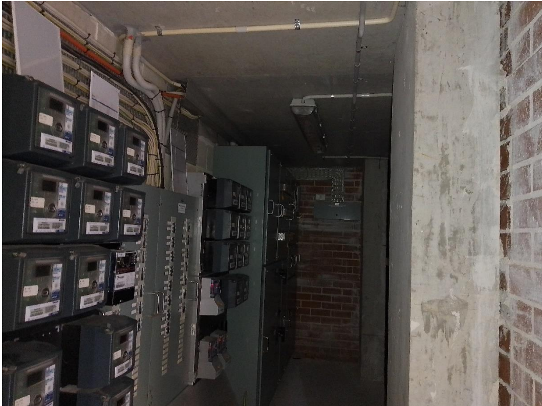
Photo 1: East wing, Main switch board room.
