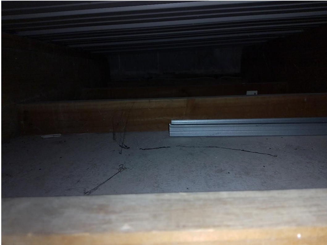
Photo 3: West wing, central laundry, above false ceiling, dust, lead detected.
