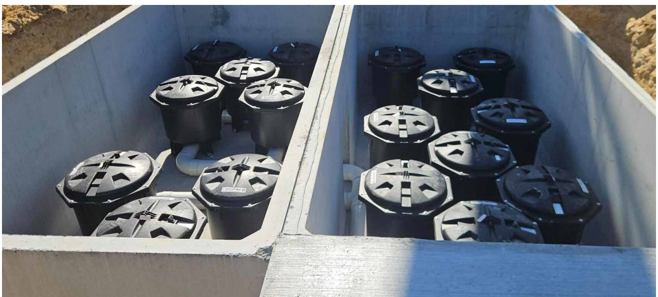
Figure 1 - AtlanFilters in a concrete chamber / vault
