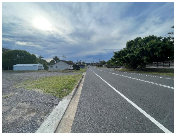
Curb and gutter off the entrance to Lot 37.
