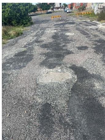
Large pothole located in the existing seal on Lot 24.
