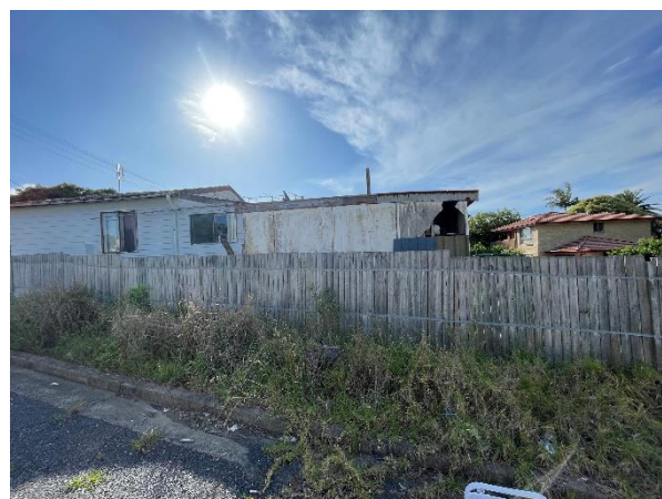
Broken wall on neighbouring site to the west, potential source of scattered building material on the site.
