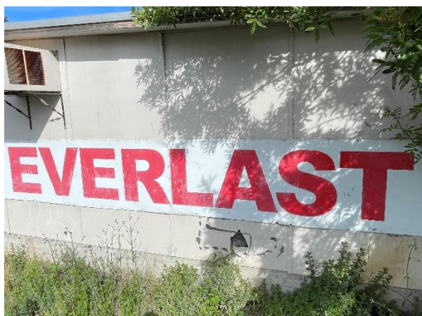
Broken wall on neighbouring site to the east, potential source of scattered building material on the site.
