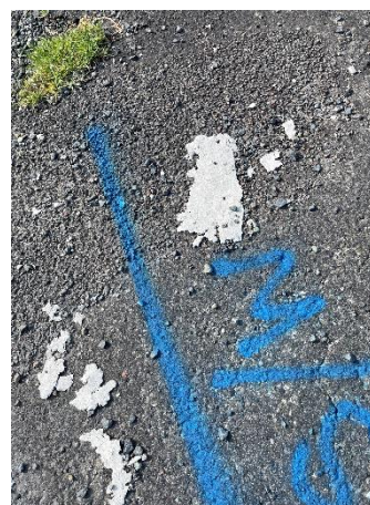
Potential ACM on surface of the site.
