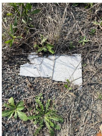
Potential ACM on surface of the site.
