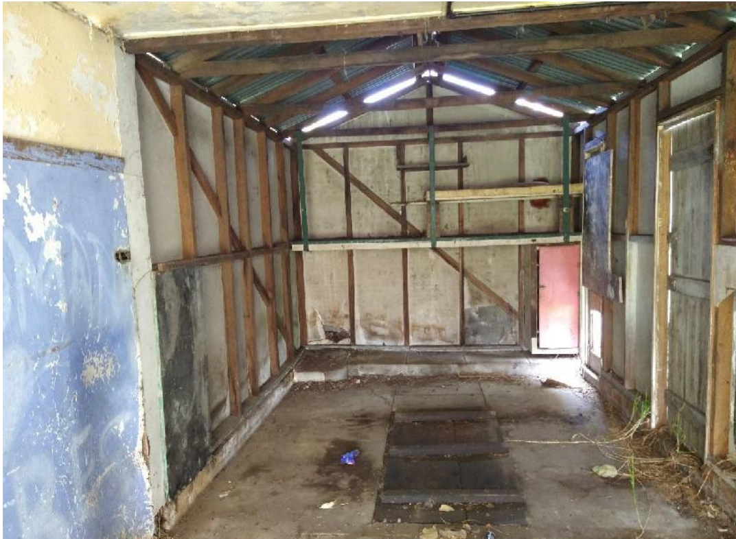
Photo 6: General view of shed structure to the rear of No. 23 Urunga Parade. Potential asbestos containing material (PACM) panels were observed on the walls.
