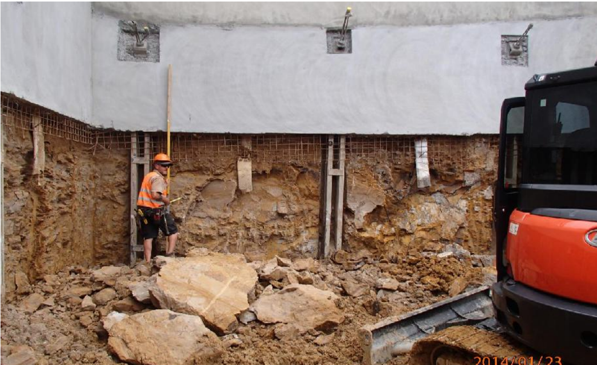
Photo 11: View looking west at a fault zone daylighting in the third bench of the Wollongong Private Hospital site adjacent to the western boundary with No. 366 Crown Street.
