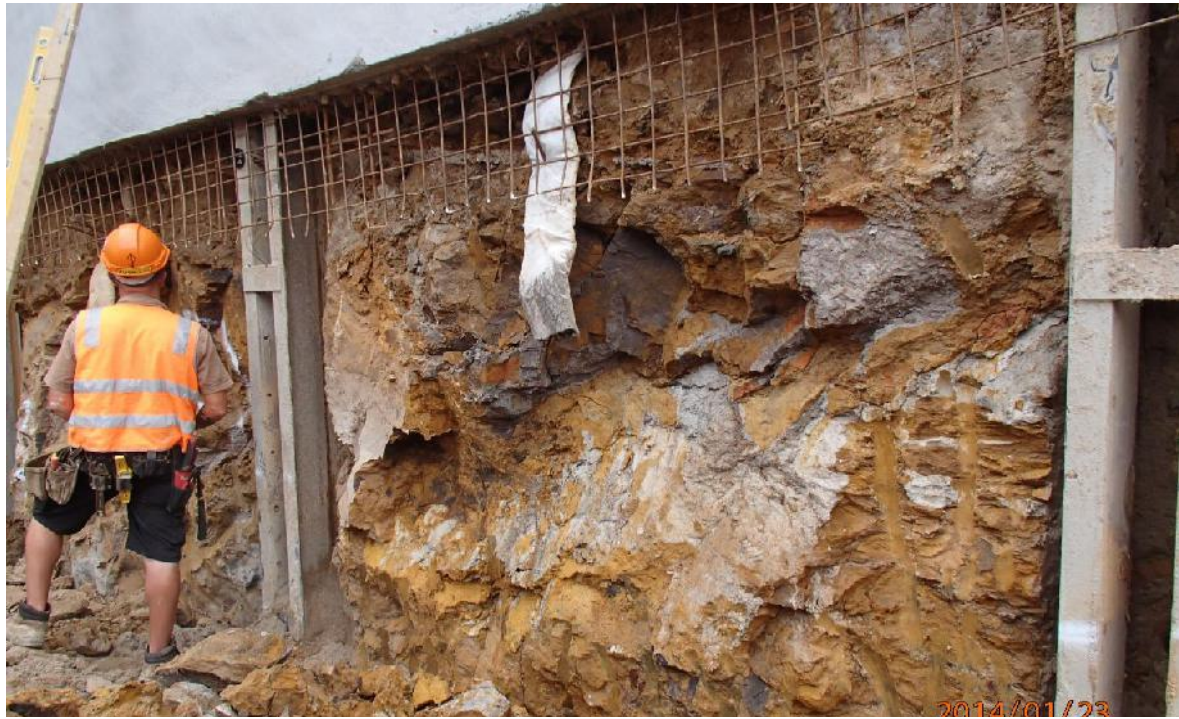
Photo 12: View looking south west at the shear surface exposed in a fault plane exposed in the third bench of the Wollongong Private Hospital adjacent to the western boundary with No. 366 Crown Street.
