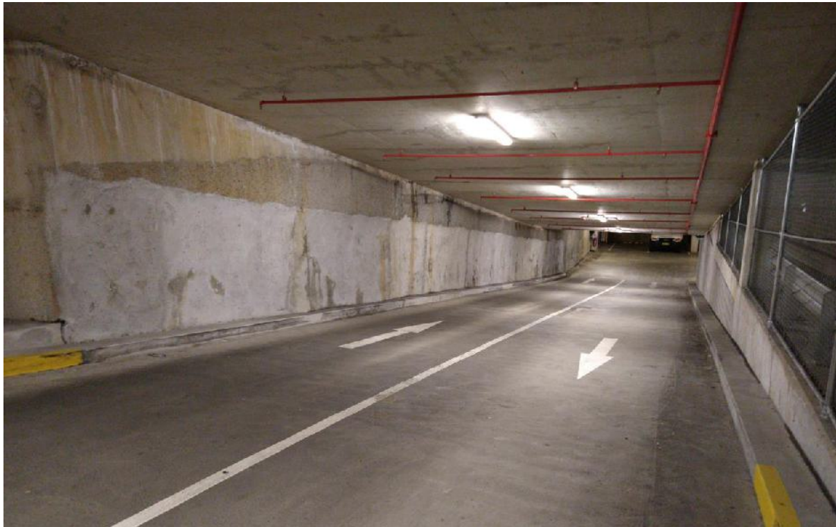
Photo 9: View looking north at the ramp connecting B1 and B2 car parks in the existing Wollongong Private Hospital basement. Note: very little seepage observed along the
