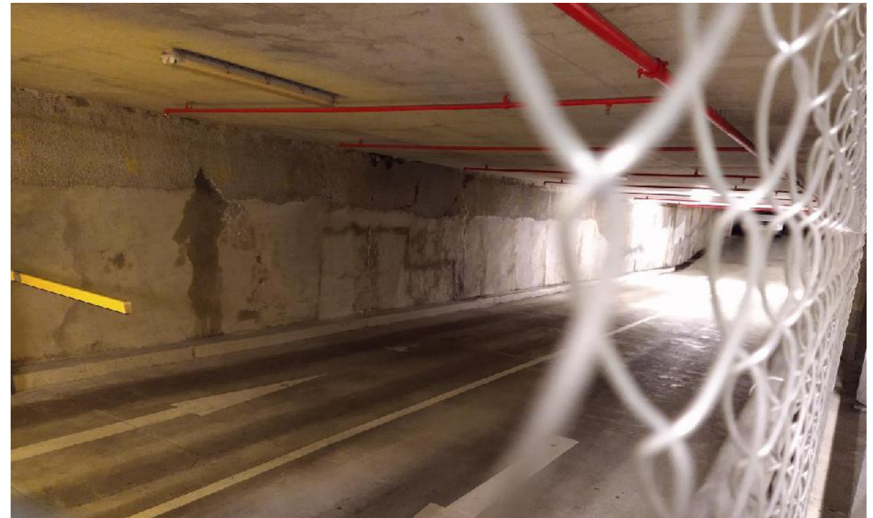
Photo 12: View looking north at the ramp connecting B2 and B3 car parks in the existing Wollongong Private Hospital basement. Note: minor seepage observed along the
