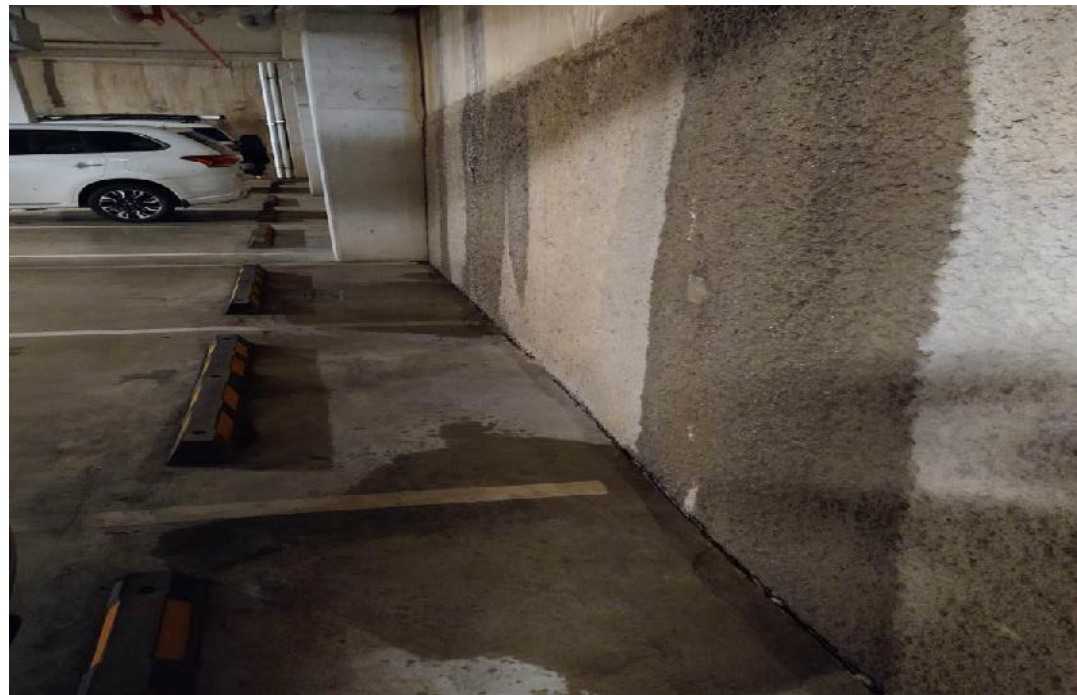
Photo 11: View looking at seepage along the northern face of the B2 car park of the existing Wollongong Private Hospital basement. Note: some splash from dripping on the adjacent
