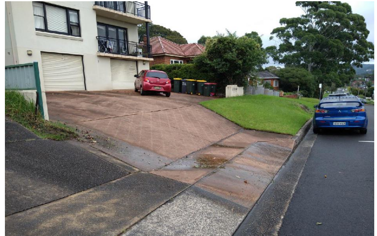
Photo 6: View looking at seepage from No. 17 Urunga Parade.
