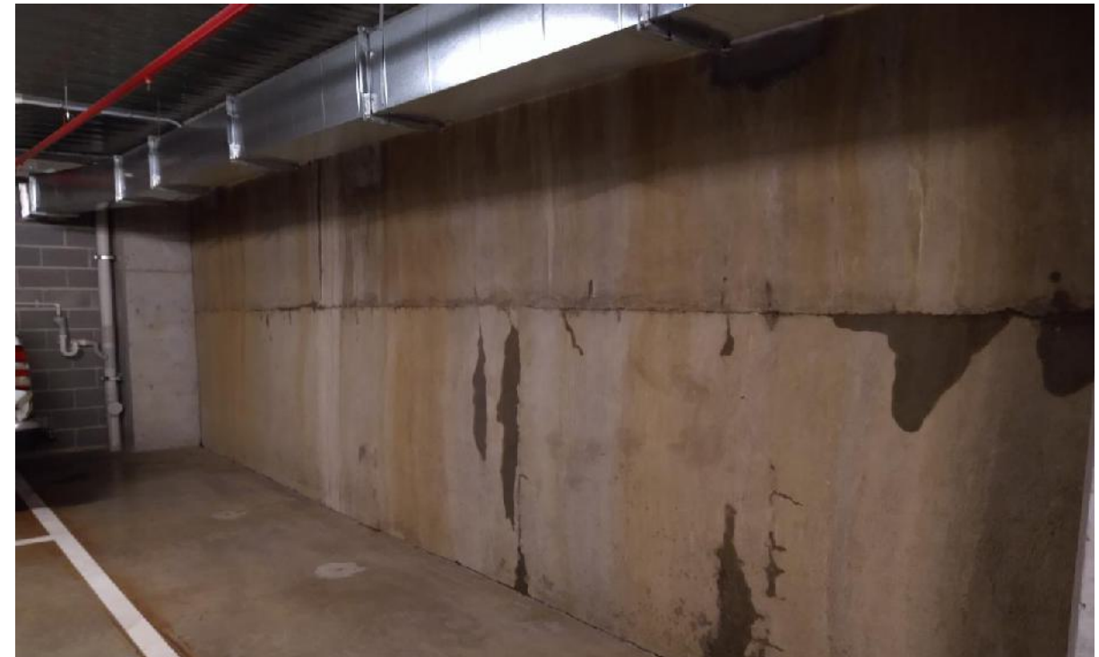
Photo 8: View looking at minor seepage in the western wall of the existing B1 car park of the Wollongong Private Hospital basement.
