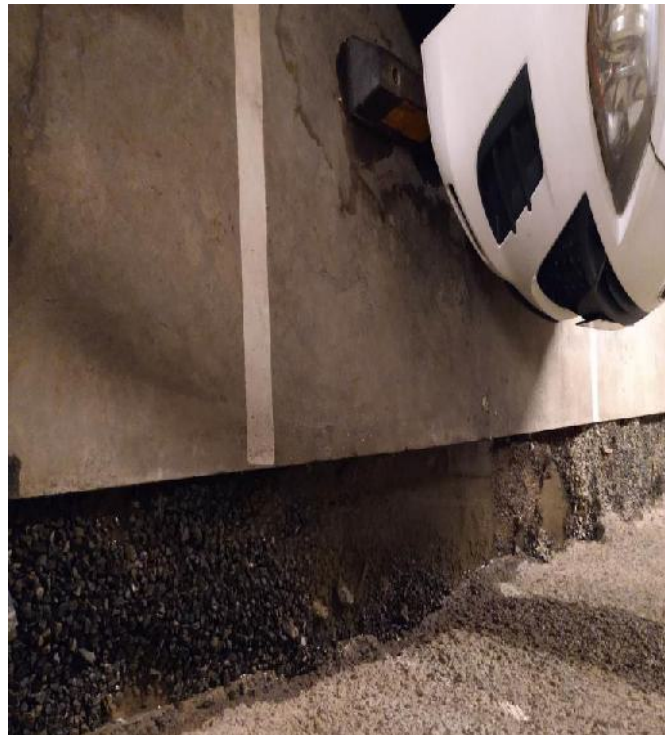
Photo 16: View looking at some water pooled in a gravel-filled drain along the northern face of the B3 car park of the existing Wollongong Private Hospital.
