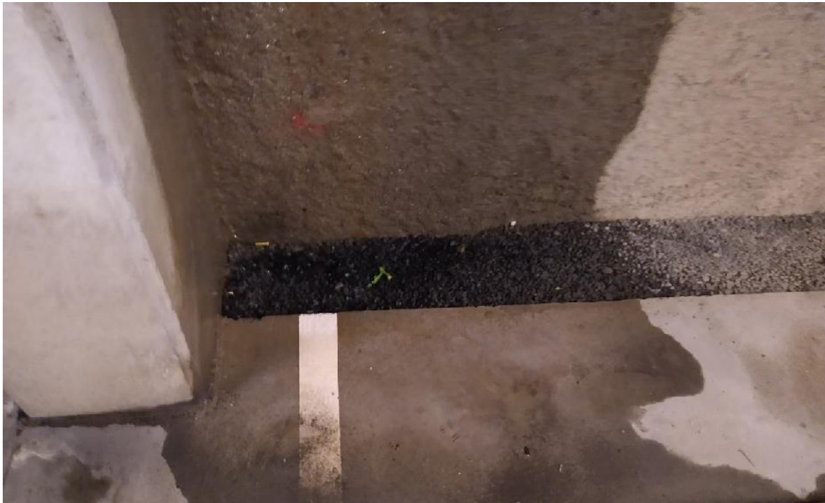
Photo 15: View looking at seepage along the northern face of the B3 car park of the existing Wollongong Private Hospital basement. Note: some splash from dripping on the adjacent slab.
