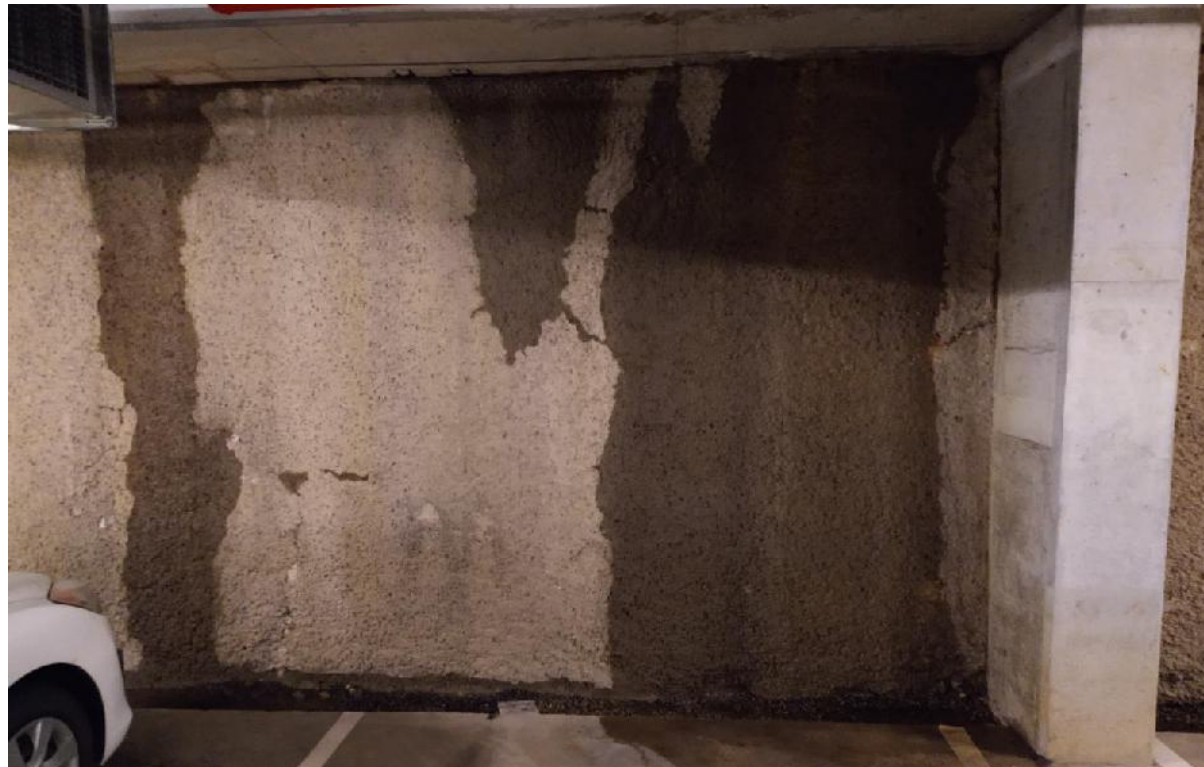
Photo 14: View looking at seepage along the northern face of the B3 car park of the existing Wollongong Private Hospital basement. Note: some splash from dripping on
