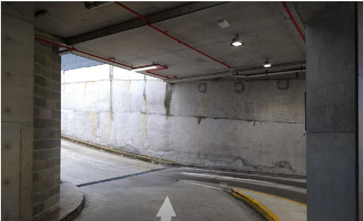
Photo 7: View looking south west at the Crown Street ramp entrance to the existing Wollongong Private Hospital B1 car park. Note: minor seepage near joins in the shotcrete.
