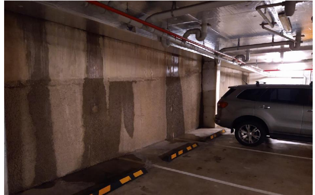
Photo 10: View looking at seepage along the northern face of the B2 car park of the existing Wollongong Private Hospital basement. Note: some splash from dripping on
