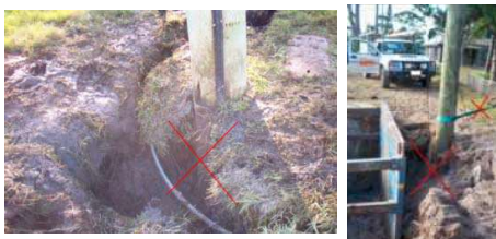
Above: Poles with become unstable if undermined
