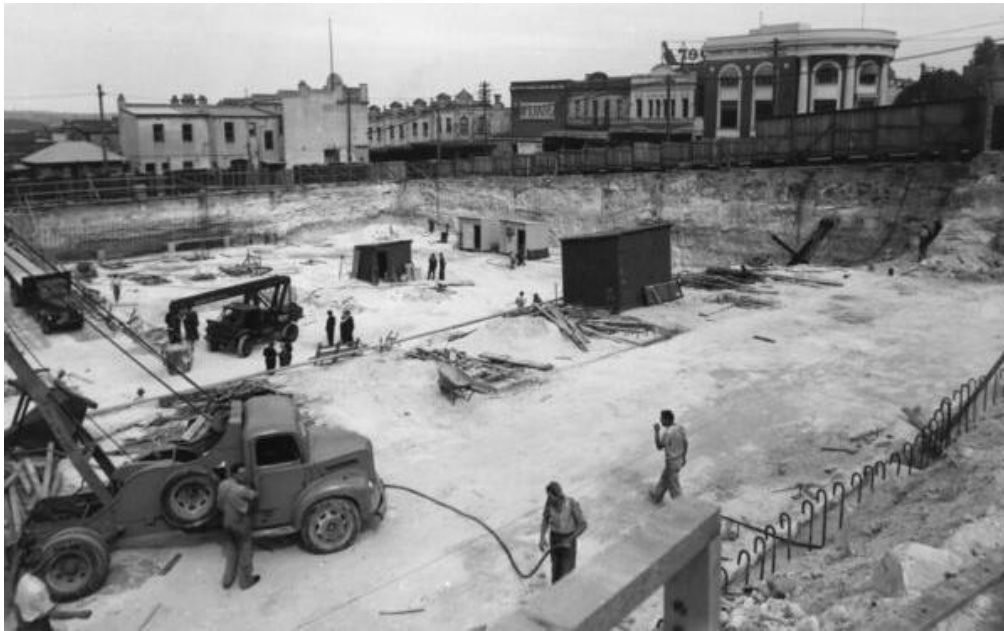
Figure 4-8: South-facing photograph showing the excavation site for 105 Miller Street as it appeared in 1955, highlighting the deep excavation undertaken, which would have significantly disturbed any soil profiles.
