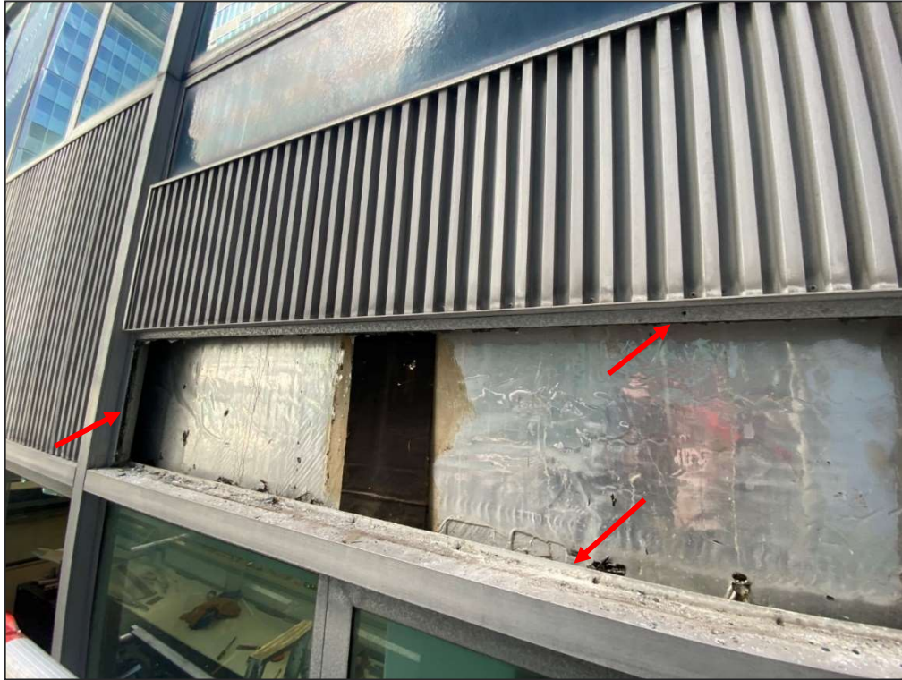
Photograph 7: The grey mastic surrounding the colour-back glass panels contain asbestos.
