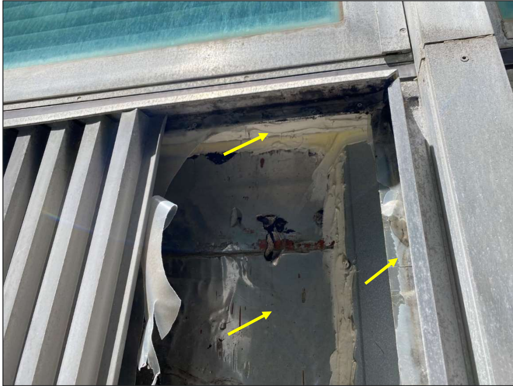
Photograph 9: As per Photo 8
