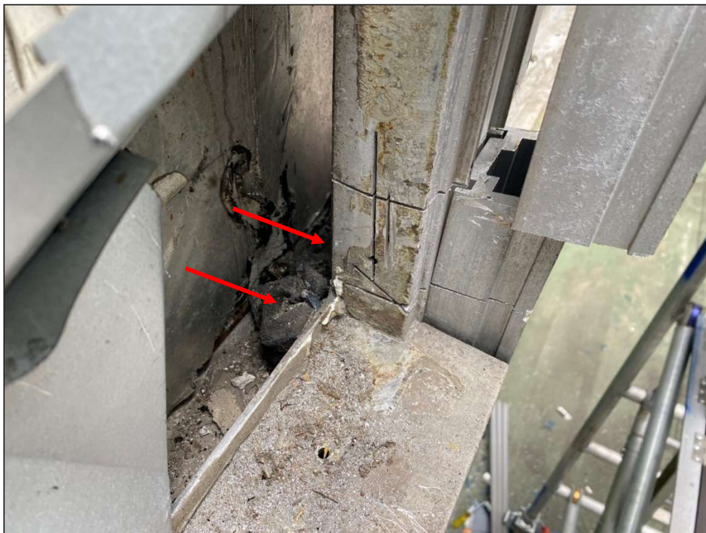
Photograph 12: The grey /brown mastic identified at the rear of the mullion / head transom connection contains asbestos.
