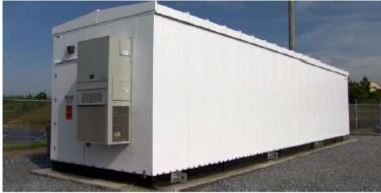
Figure 7: Typical 40 ft modified shipping container for battery energy storage (extracted from Edify Memo)
