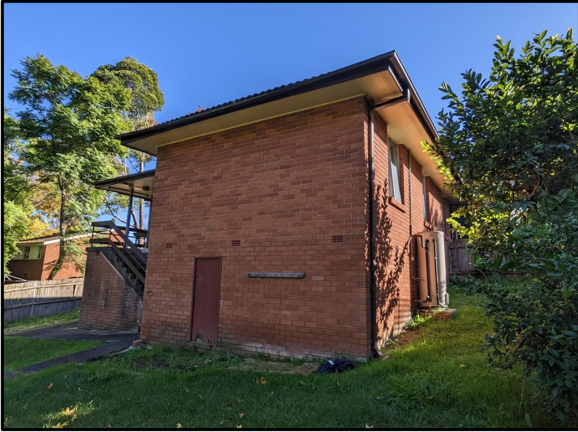
Figure 20. Rear view of the brick dwelling within the property at No. 15B Moseley Street.
