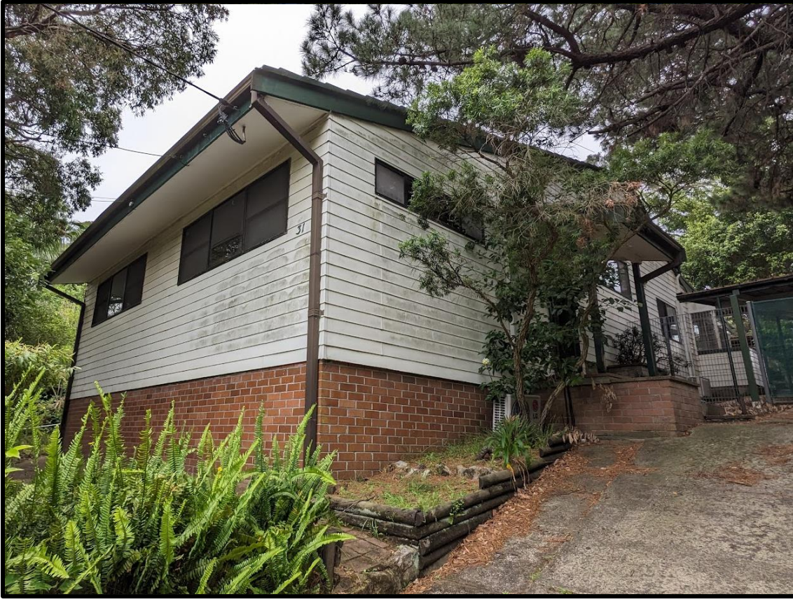
Figure 14. Rear view of the dwelling within the property at No. 31 Donald Street.
