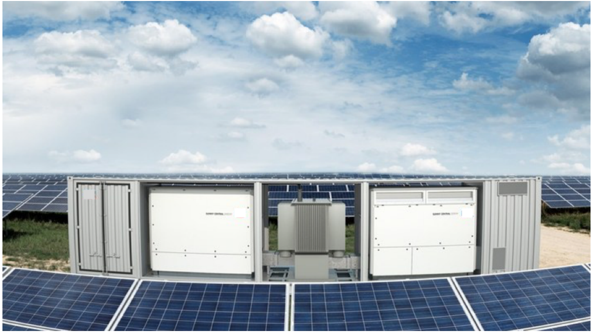
Figure 19: Example of containerised inverter rooms deployed in a solar field
