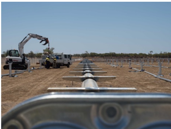
Row of installed trackers with panel brackets
