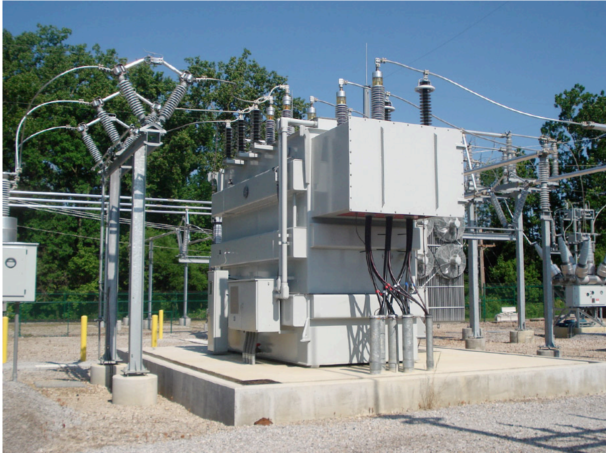
Figure 18: Example of substation
