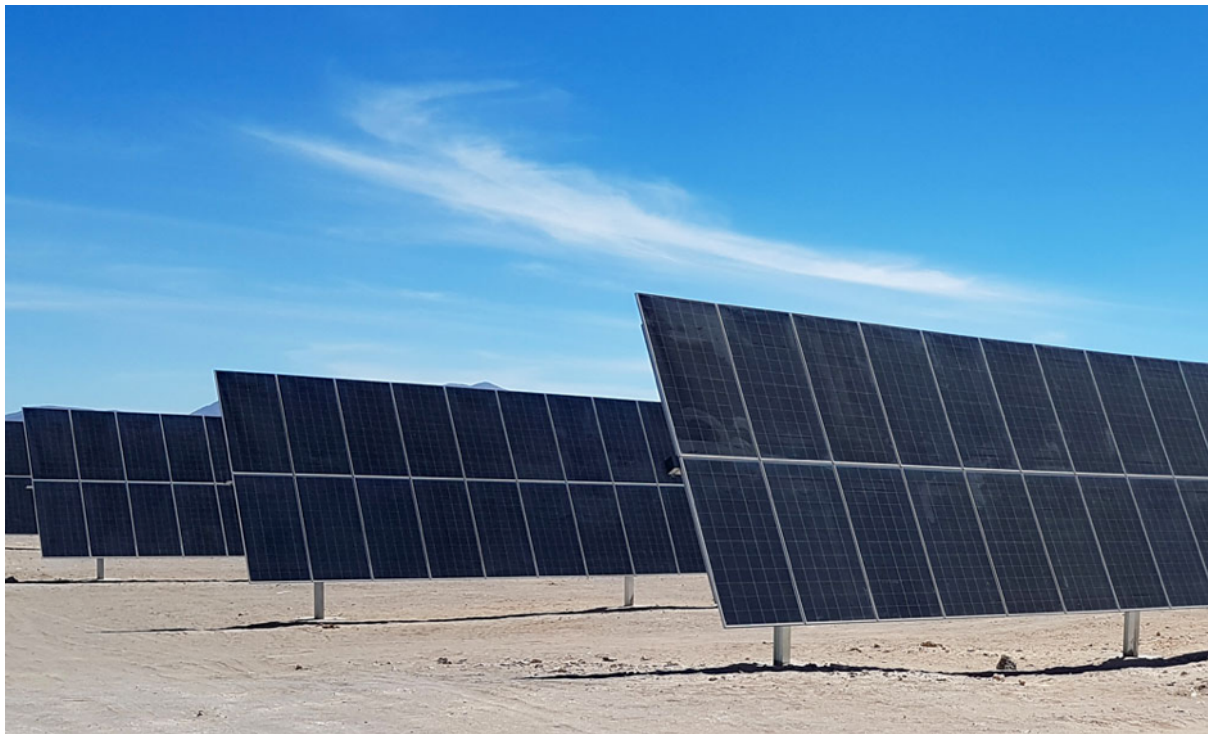
Figure 14: Example of installed double portrait single axis tracking solar PV installations
