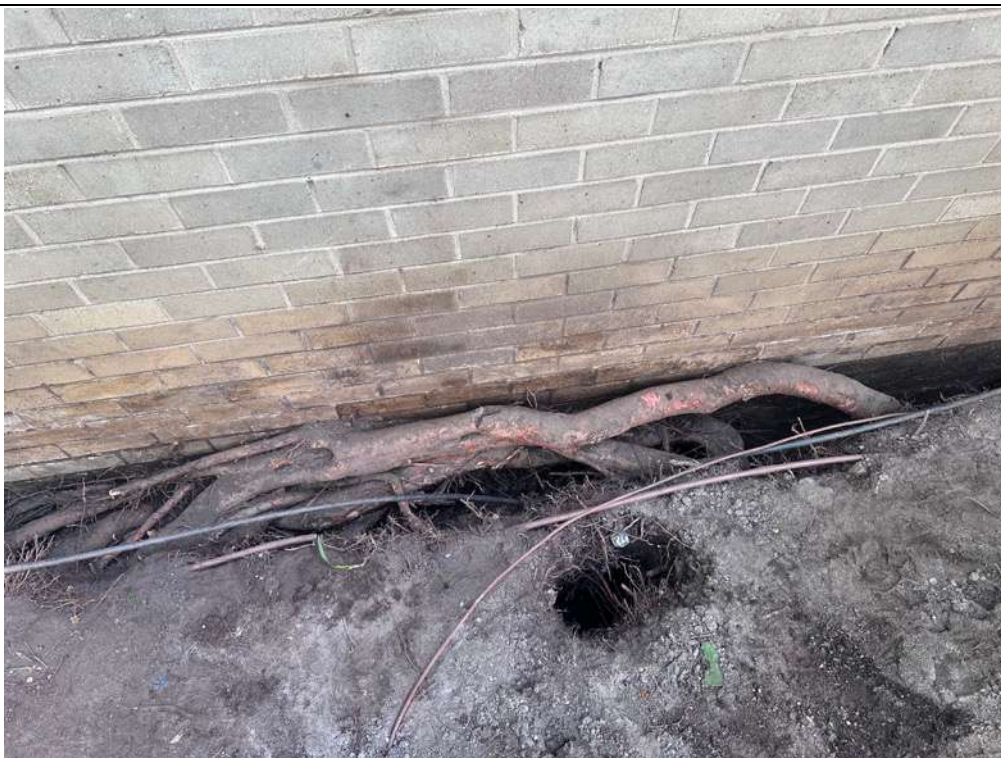
Image 6: Root 2-5, which grow in a bundle adjacent to the existing building footing.
