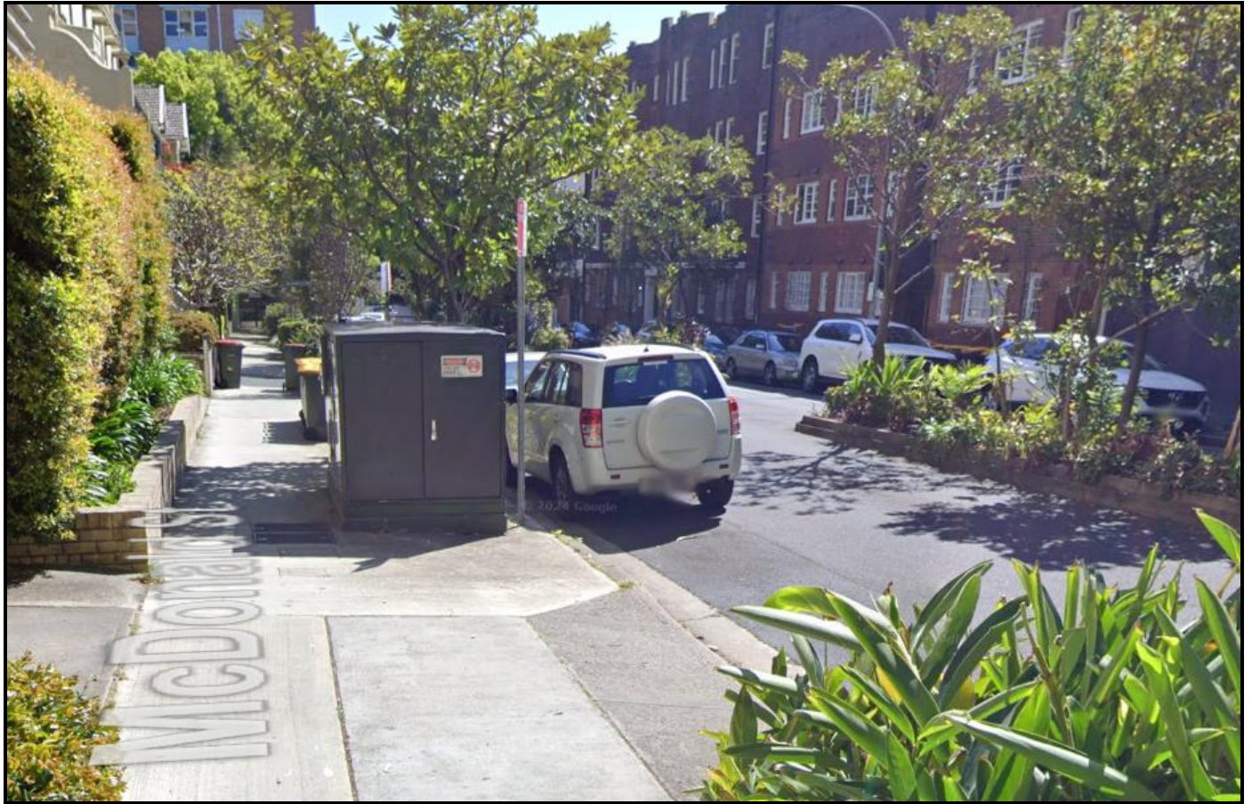
Figure 3: Existing Kiosk Substation on McDonald St
