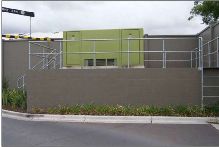
Figure 51 - Example substation raised above 1:100 flood level
