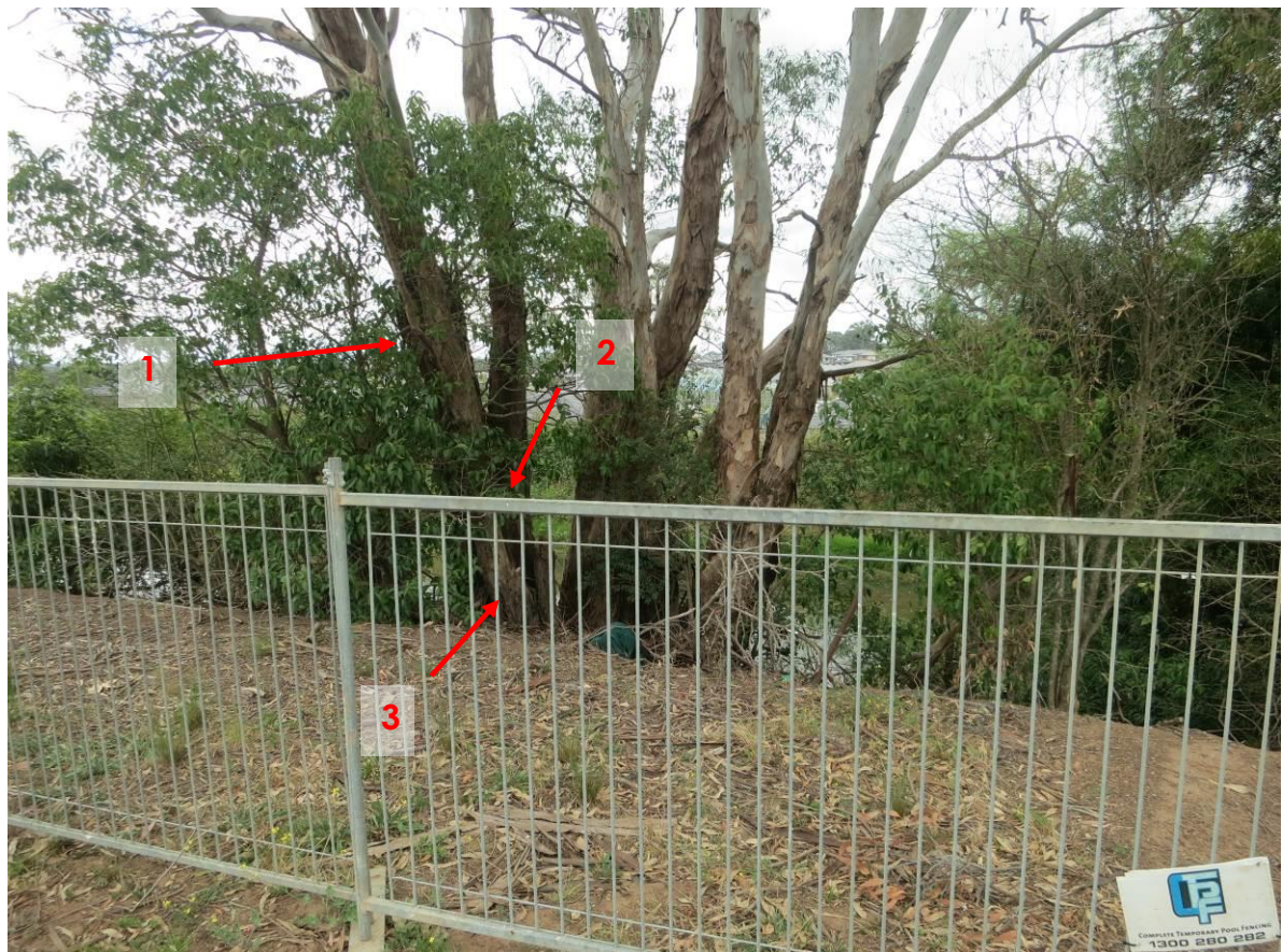
Image 4 – Photo taken from south-east, showing location of structural defects (1, 2 & 3)
