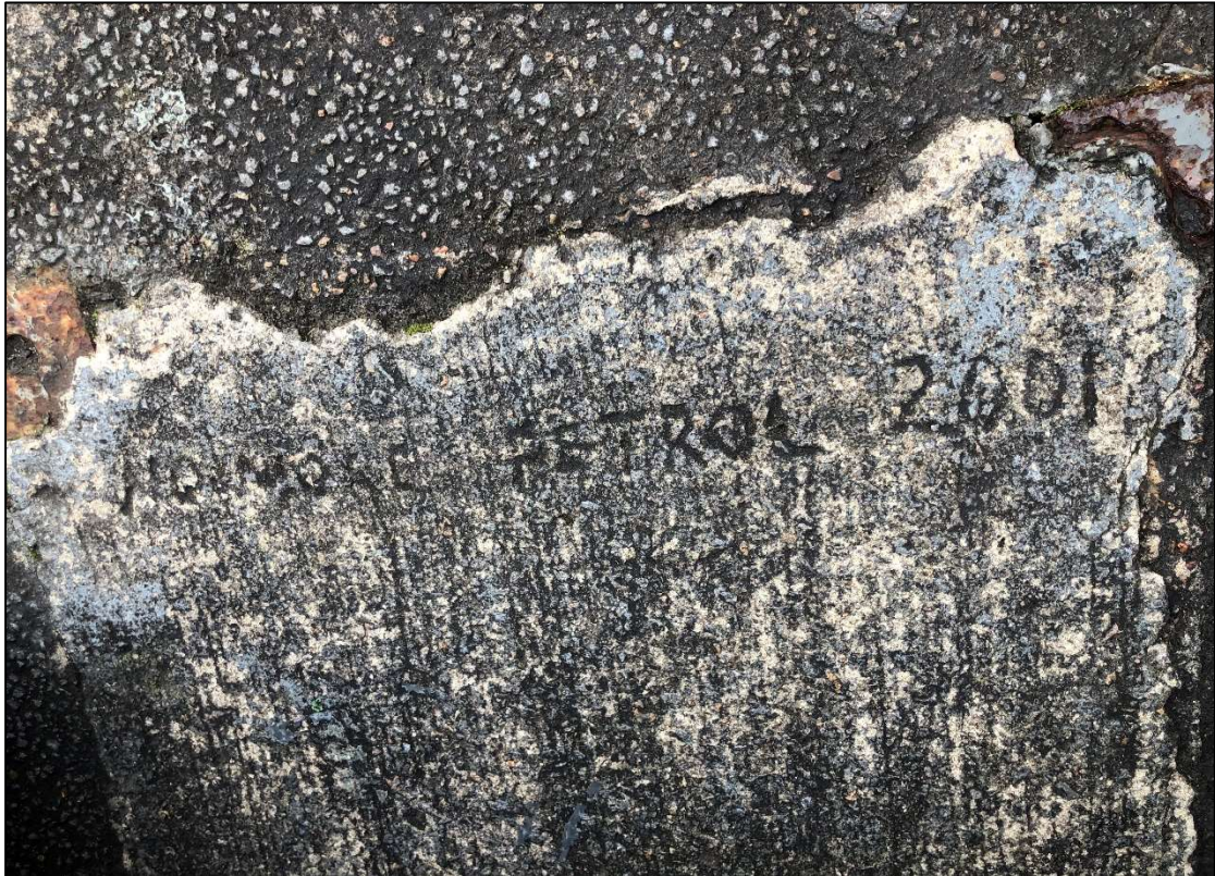
Photo 23: Marked concrete patch, Lot B
