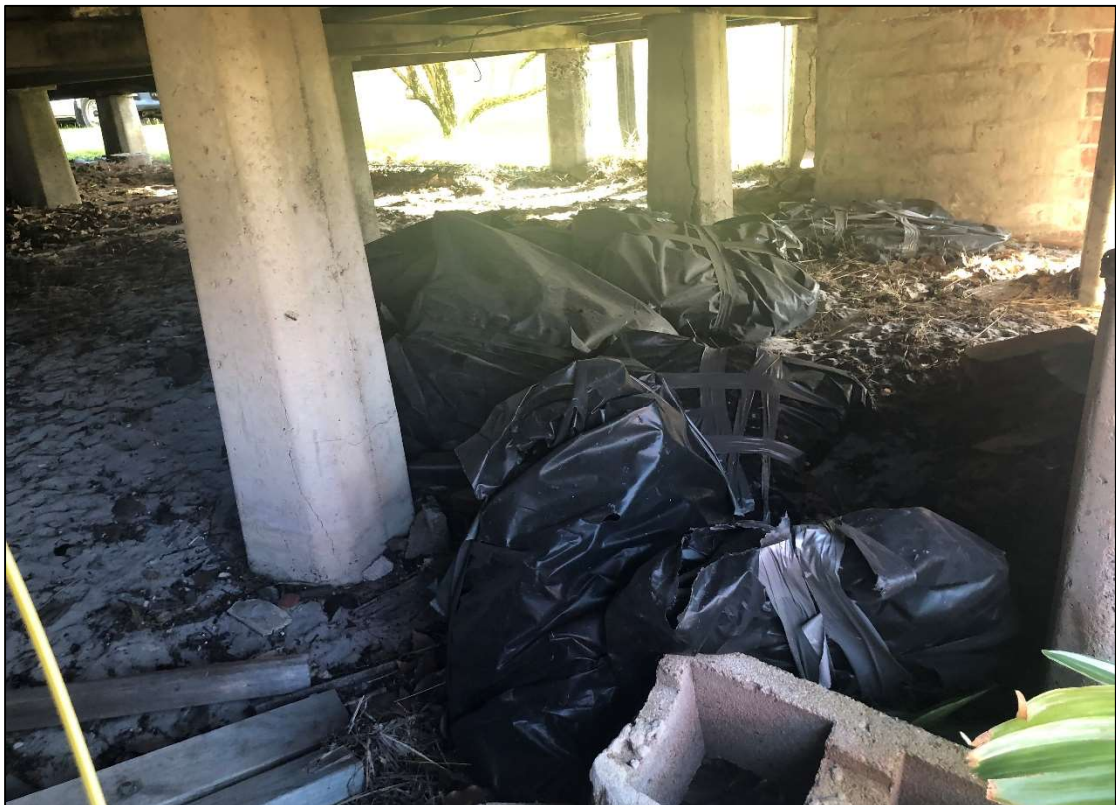
Photo 8: Fibro sheeting in black plastic, subfloor of residential dwelling (Lot 15), looking west
