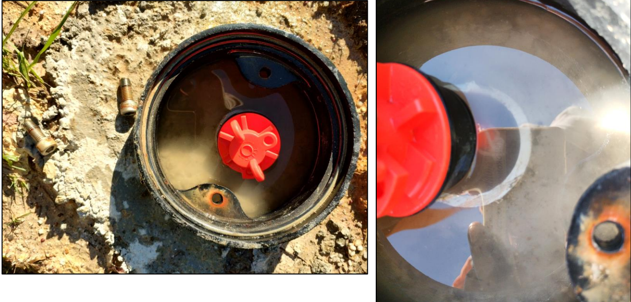
Figure 7: Groundwater at surface of monitoring well at Bore 109A (7 May 2025)
