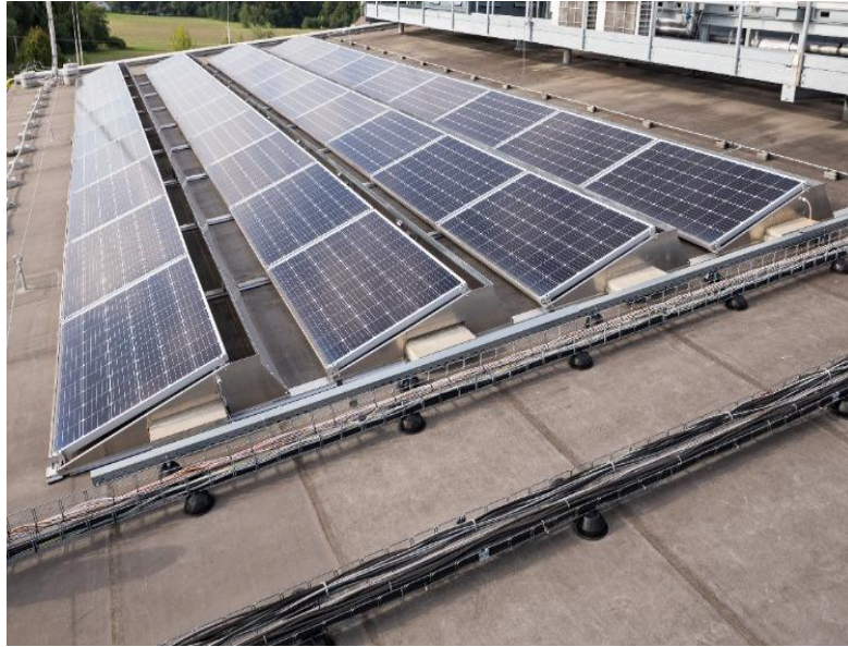
Figure 4 Example of rooftop solar installation
