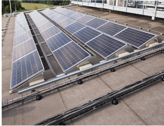
Figure 11 Example of rooftop solar installation
