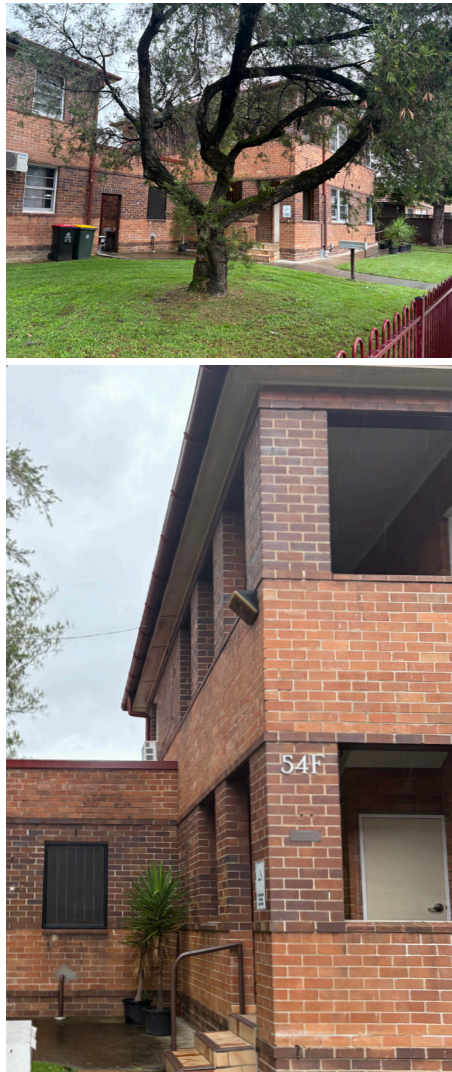
Existing trees and building bricks
