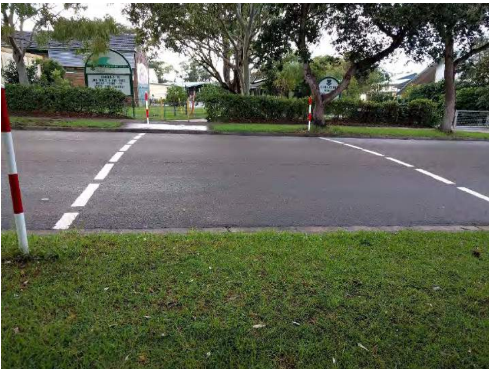
View of Children's Crossing on Playfair Road with no kerb ramps
