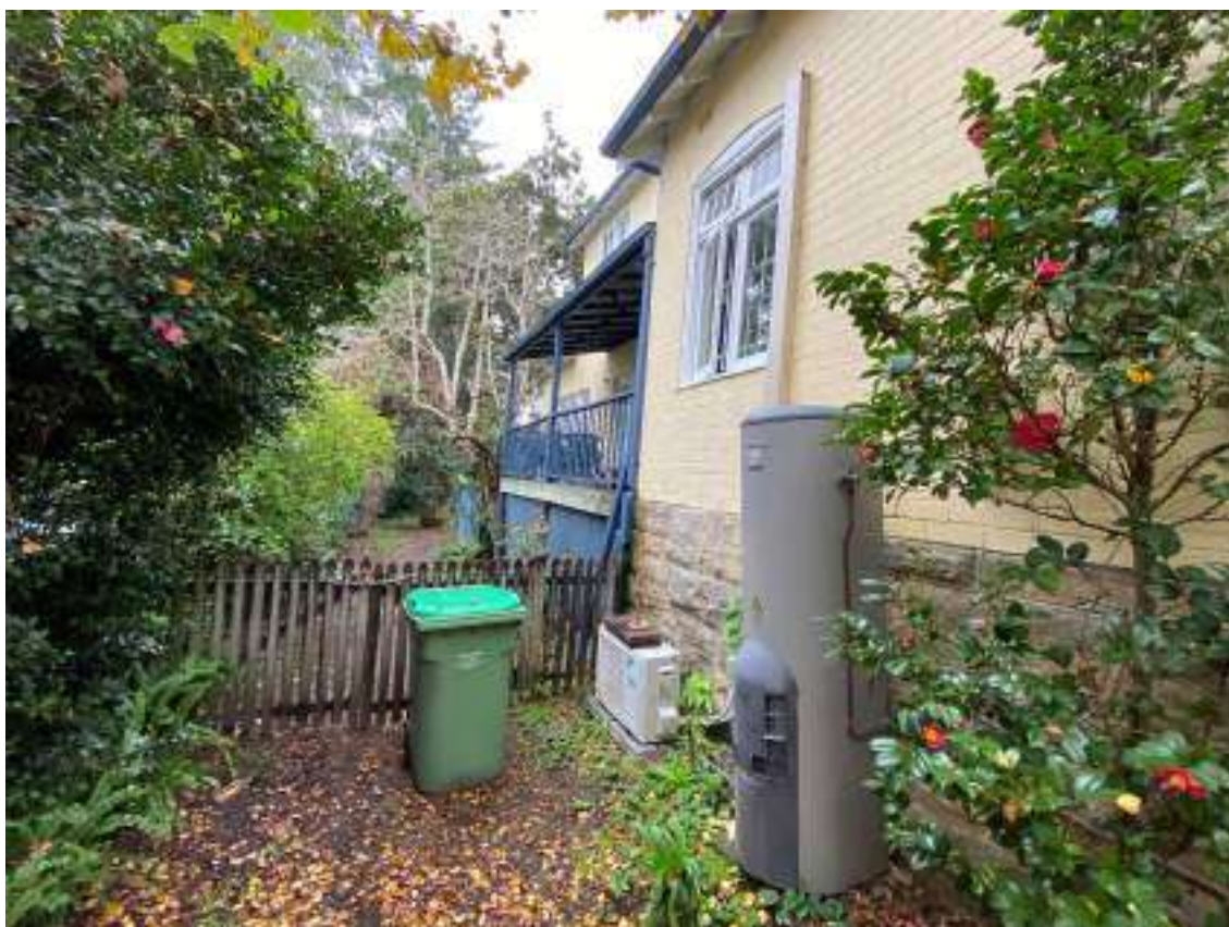
Photograph 13 - Suspended footing and stone foundation in fair condition, AC unit and water tank were found next to the eastern wall of the property (17 Middle Harbour Road)
