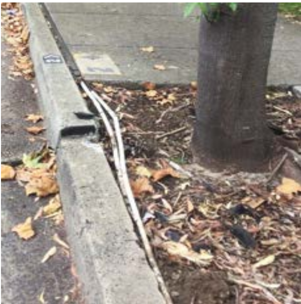
Figure 5: cable housed in white conduit
