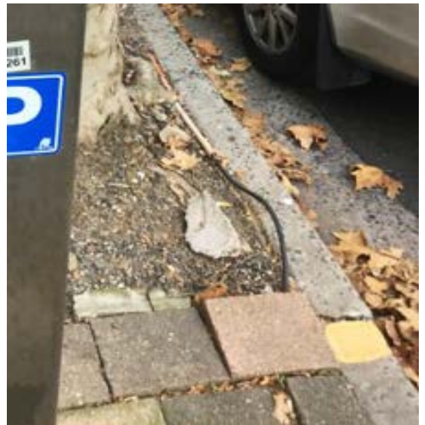
Figure 6: black cable housed in orange conduit
