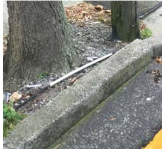
Figure 4: black cable housed in white conduit
