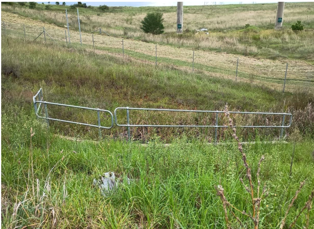
Photograph 8: Stormwater System at Service Alignment Chainage 560 m
