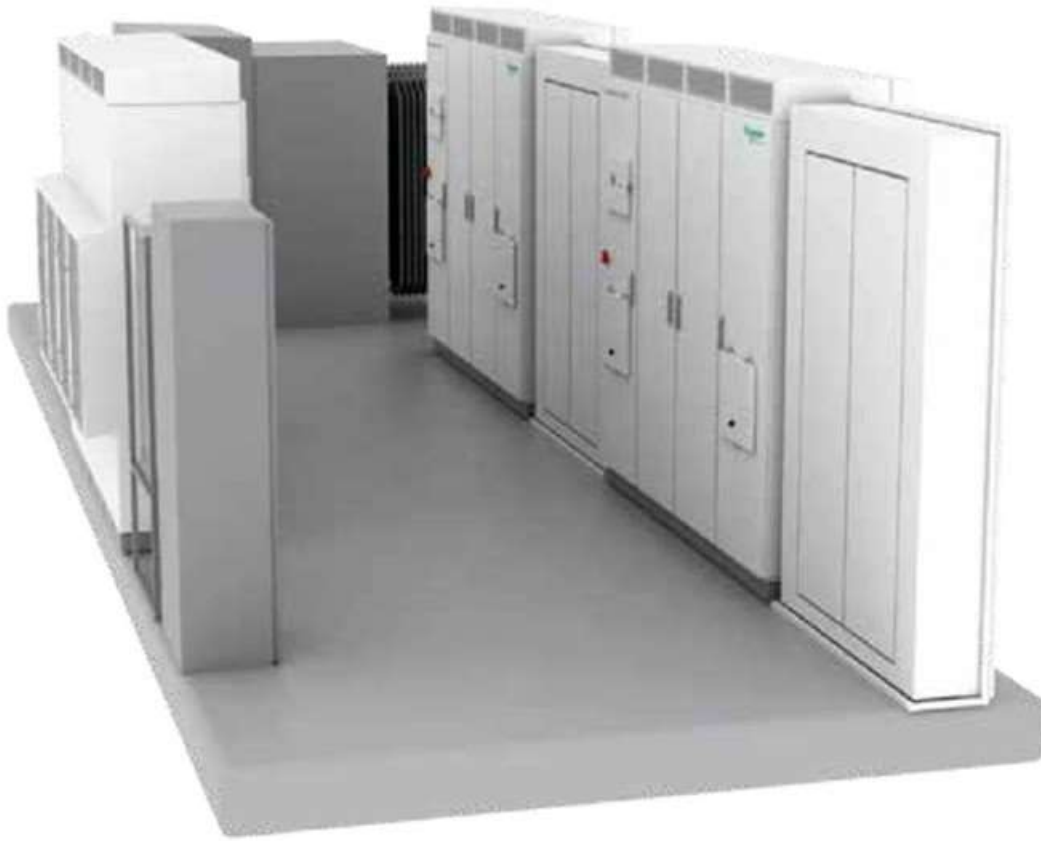
Figure 3-10 Example of a PV skid
